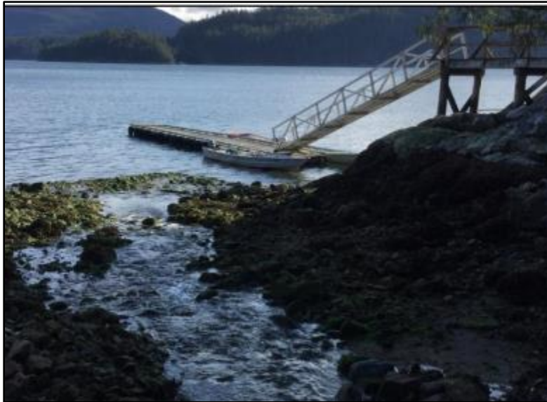
Figure 2: Southeastern view of the existing Hoskyn Channel Landing Facility. A stream flows from the north towards the dock at low tide has since been redirected slightly away from the dock.
