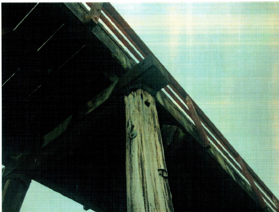
Photo 21 – Hole in Pile 9A
