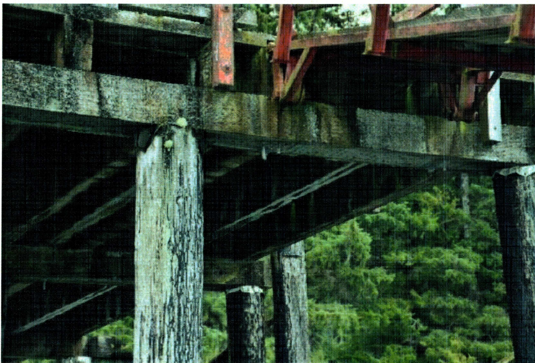
Photo 24 – Moss growth in Pile 15B
