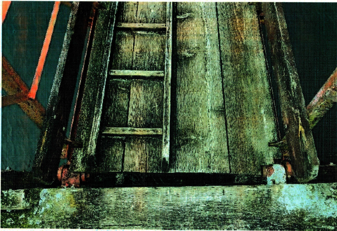
Photo 31 – Gangway Upper Hinge Connection
