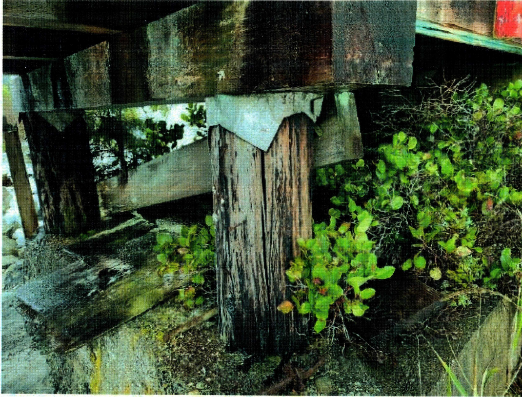
Photo 15 – Split in Pile 2A
