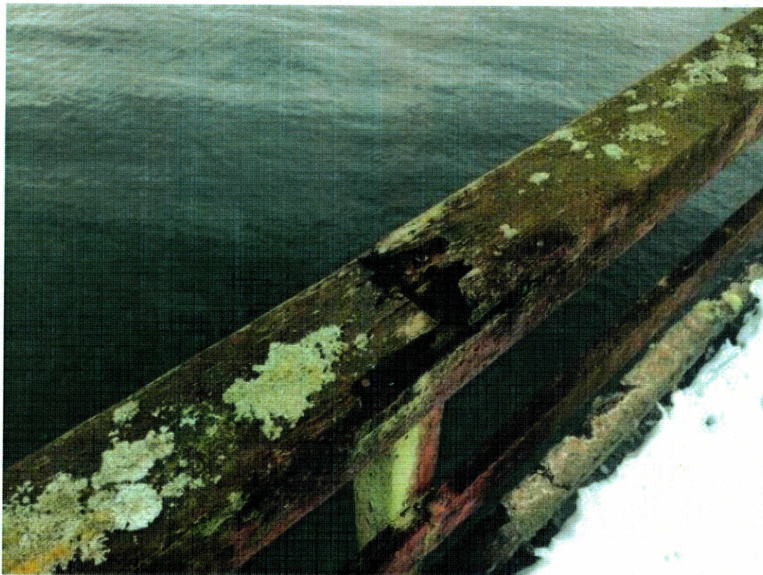
Photo 8 – Handrail deterioration between piles 11A and 12A
