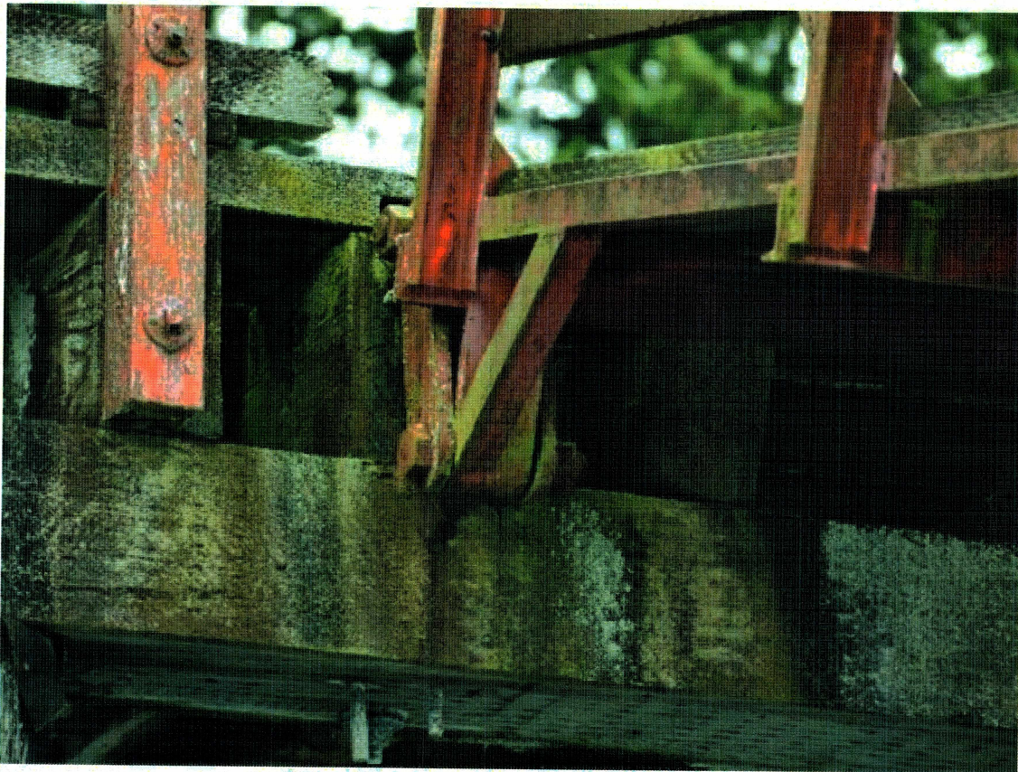
Photo 32 – Gangway Upper Hinge Connection
