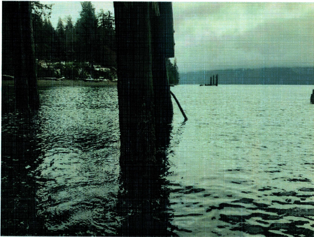
Photo 28 – Fender Pile 15C
