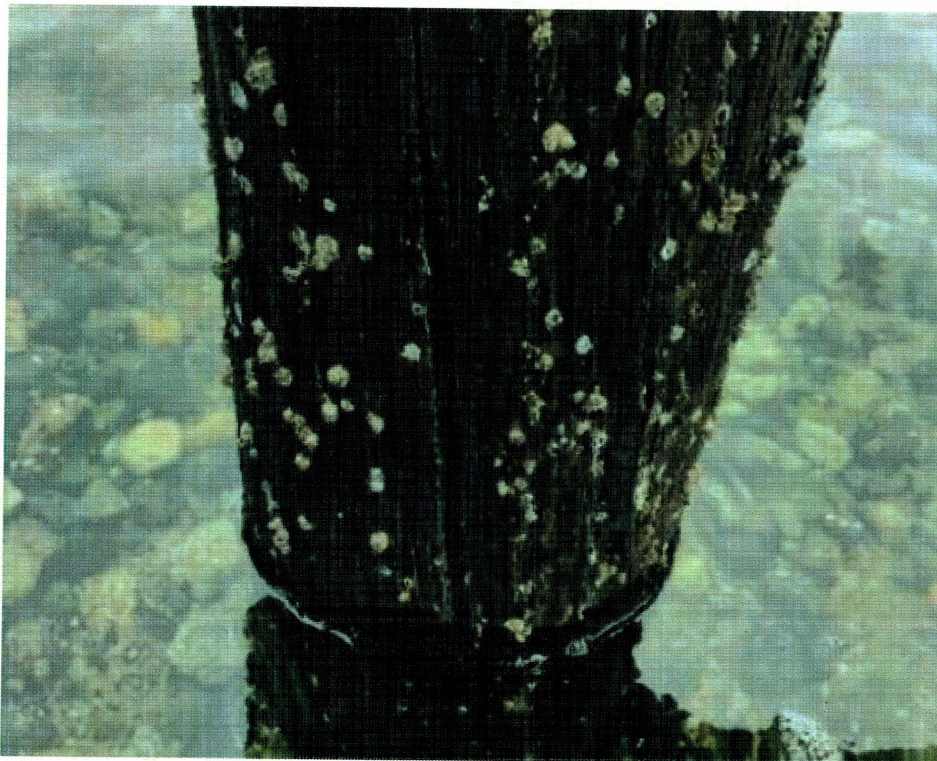
Photo 18 – Split in Pile 5A
