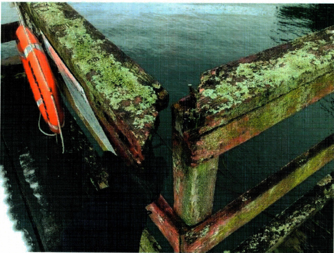
Photo 10 – Handrail deterioration between piles 14B and 14C
