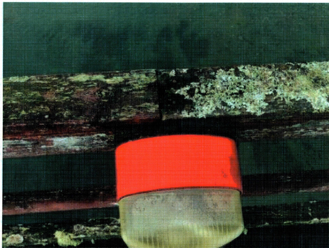
Photo 6 – Handrail deterioration between piles 8B and 9B
