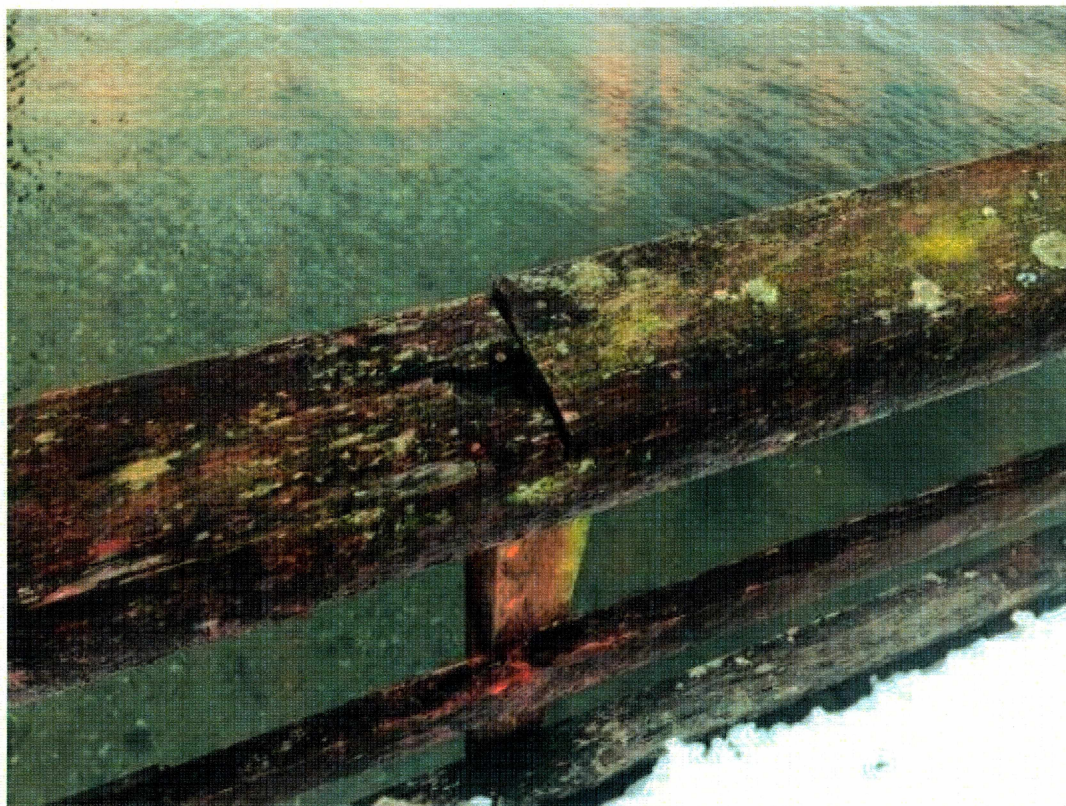
Photo 5 – Handrail deterioration between piles 7A and 8A
