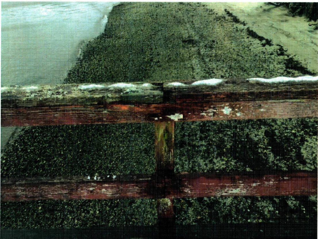
Photo 4 – Handrail deterioration between piles 4B and 5B
