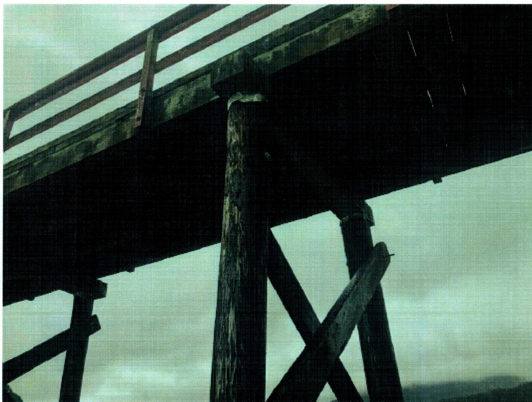
Photo 22 – Small split in Pile 10A
