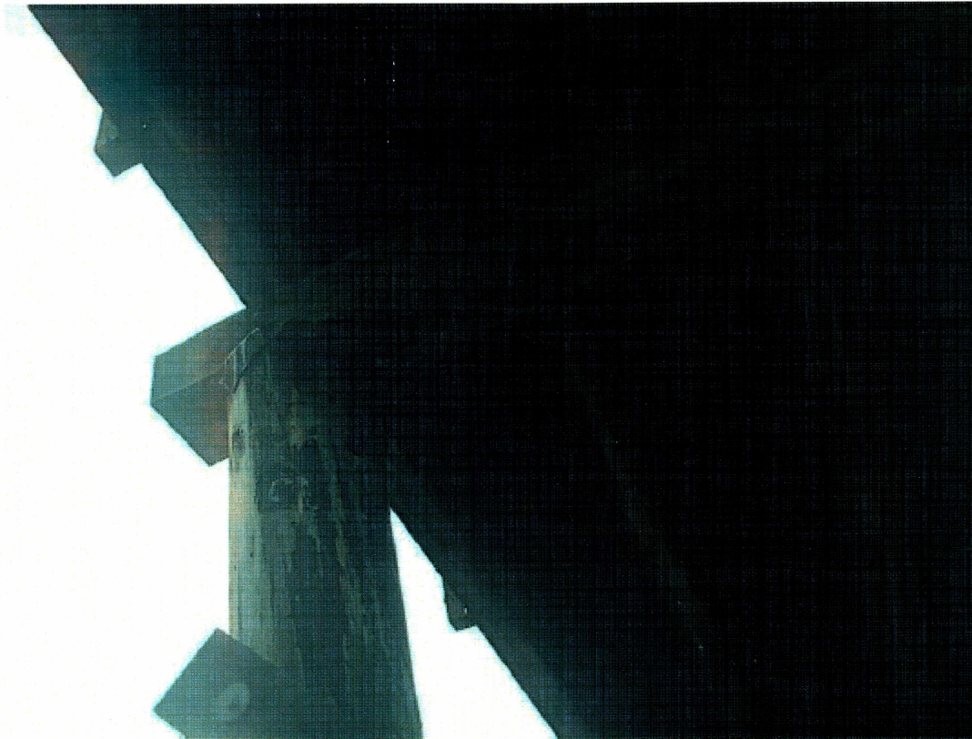
Photo 23 – Hole in Pile 12A
