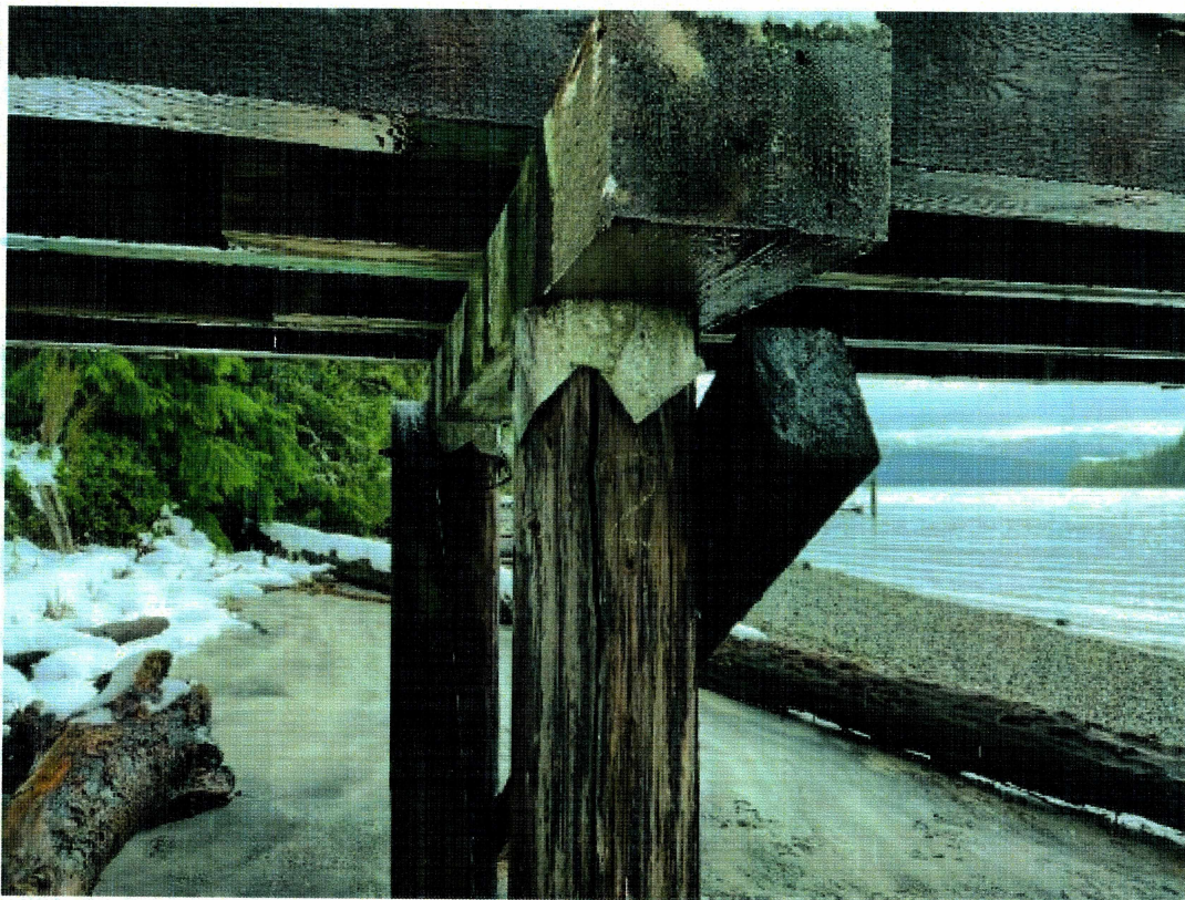
Photo 16 – Split in Pile 3B
