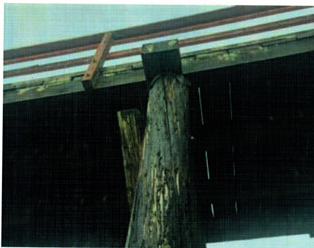
Photo 20 – Split in Pile 8A
