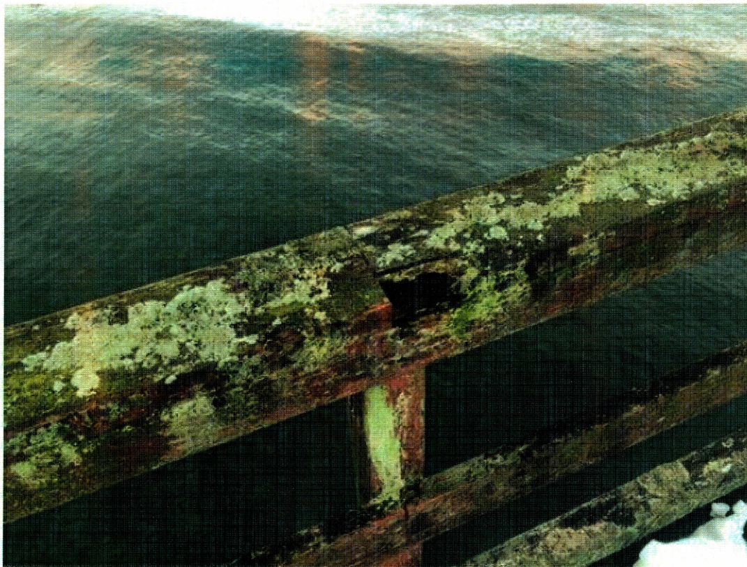
Photo 9 – Handrail deterioration between piles 12A and 13A
