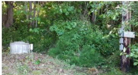
Packer’s Spring new well casing and Hydro pole
