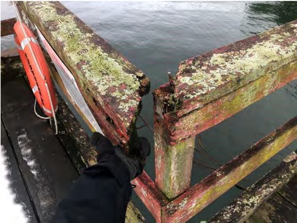
Photo 10 – Handrail deterioration between piles 14B and 14C
