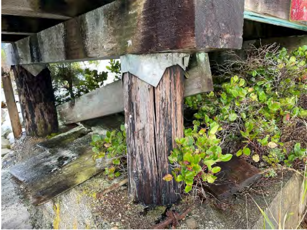
Photo 15 – Split in Pile 2A
