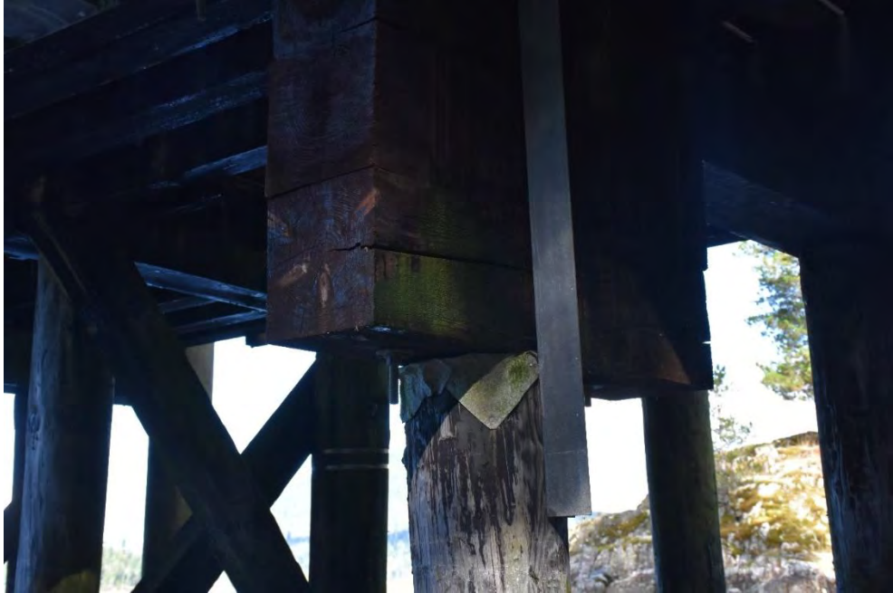
Photo 17 - Split in corbel at Bent 7
