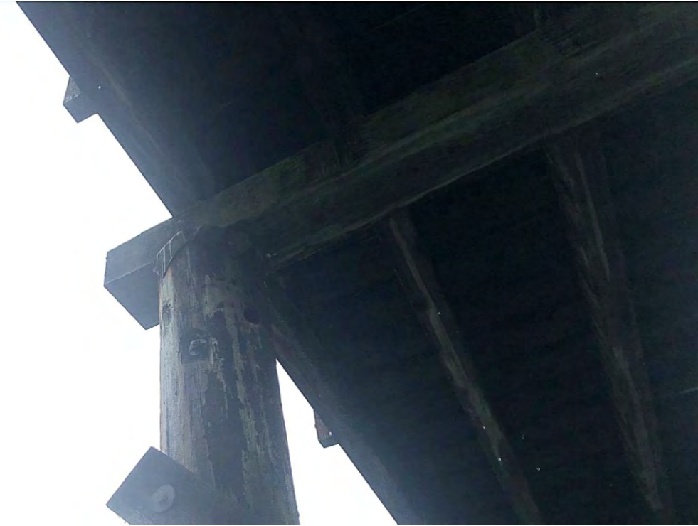
Photo 23 – Hole in Pile 12A
