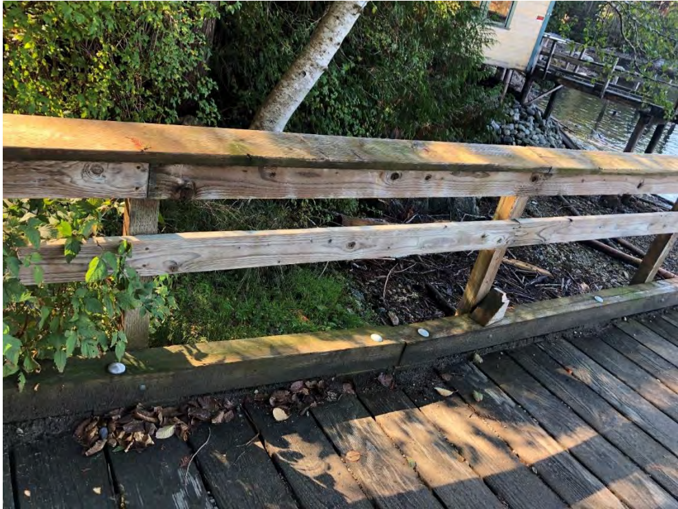
Photo 5 - Missing lower mid-rail
