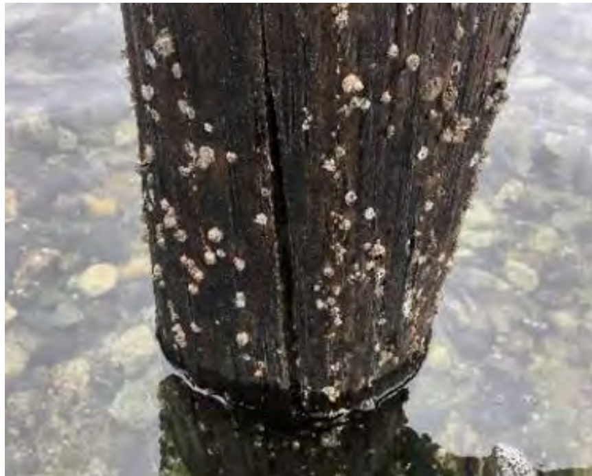
Photo 18 – Split in Pile 5A
