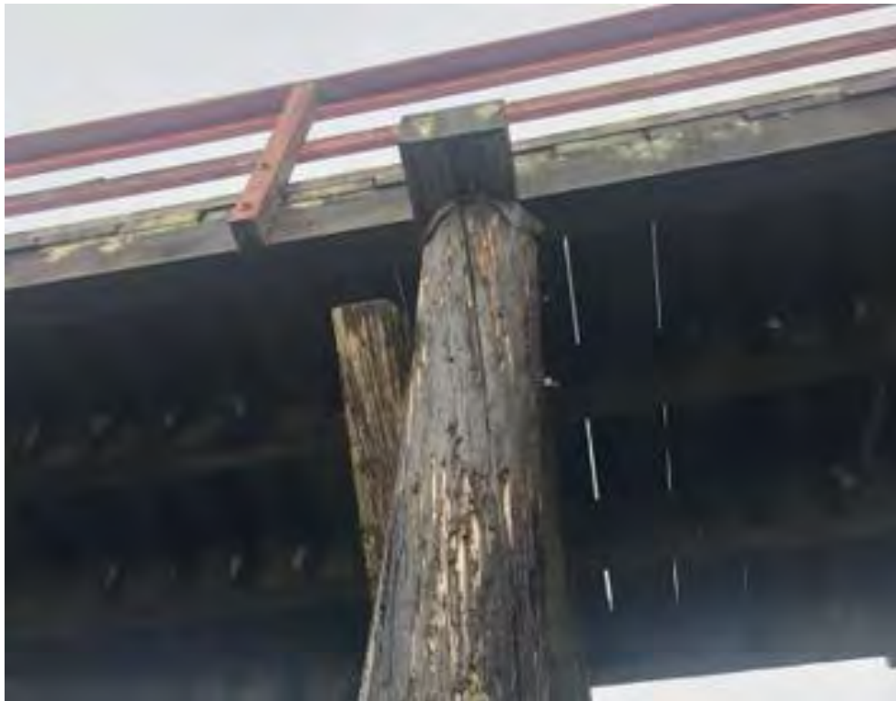
Photo 20 – Split in Pile 8A
