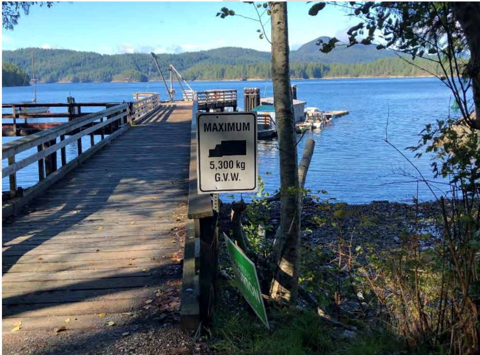
Photo 2 - Load rating sign
