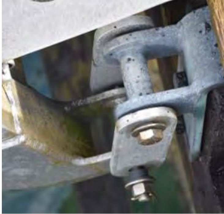
Photo 23 - Gangway Upper Hinge Connection with loose bolt
