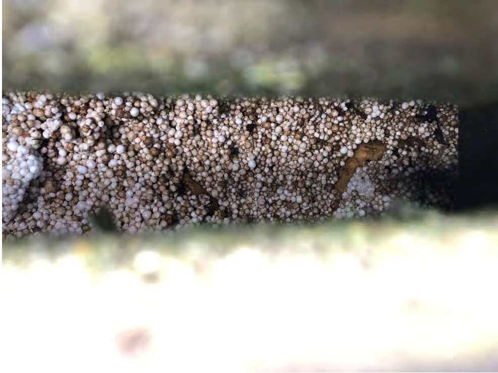
Photo 33 - Condition of exposed uncoated styrofoam billets
