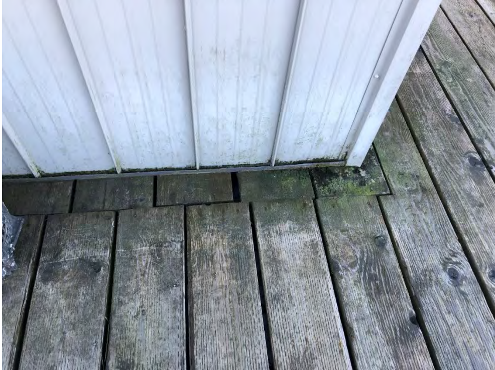
Photo 45 - Typical condition of the deck beneath the postal shed
