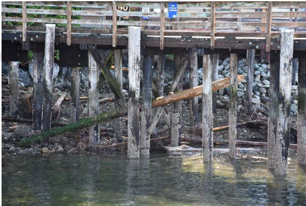
Photo 30 - North end fender piles and log debris
