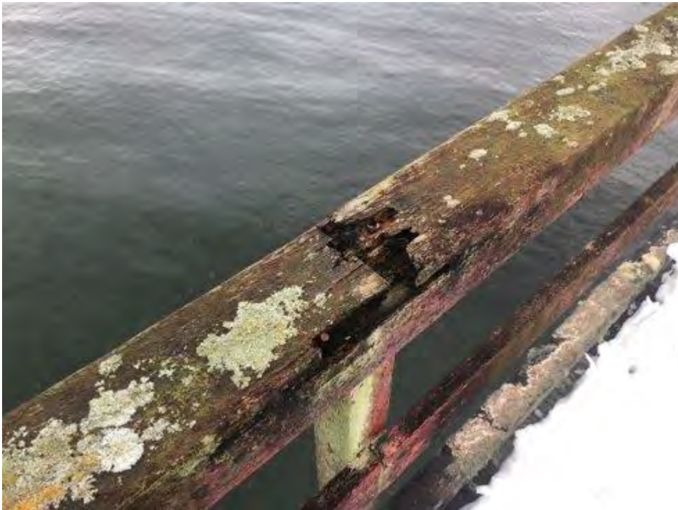
Photo 8 – Handrail deterioration between piles 11A and 12A
