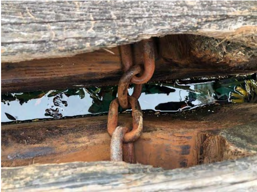
Photo 40 – Chain Connection to Float B
