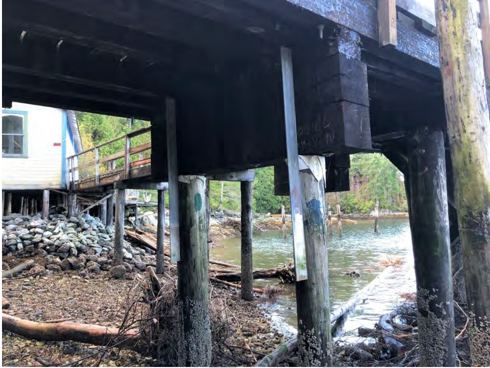
Photo 15 - Split in corbel at Bent 6
