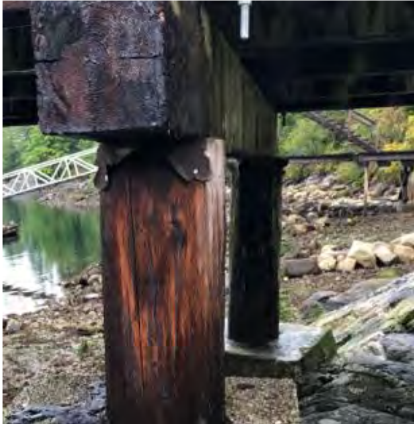
Photo 17 - Minor splitting on Pile 4B
