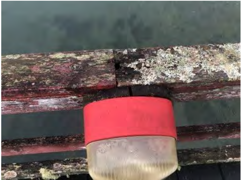
Photo 6 – Handrail deterioration between piles 8B and 9B
