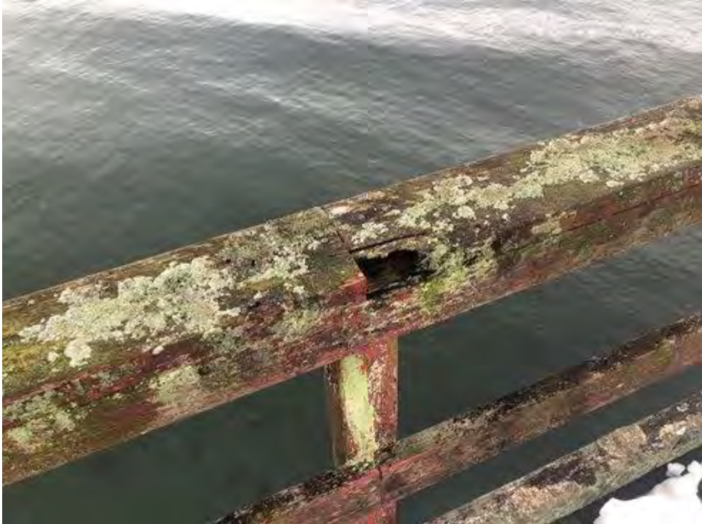
Photo 9 – Handrail deterioration between piles 12A and 13A
