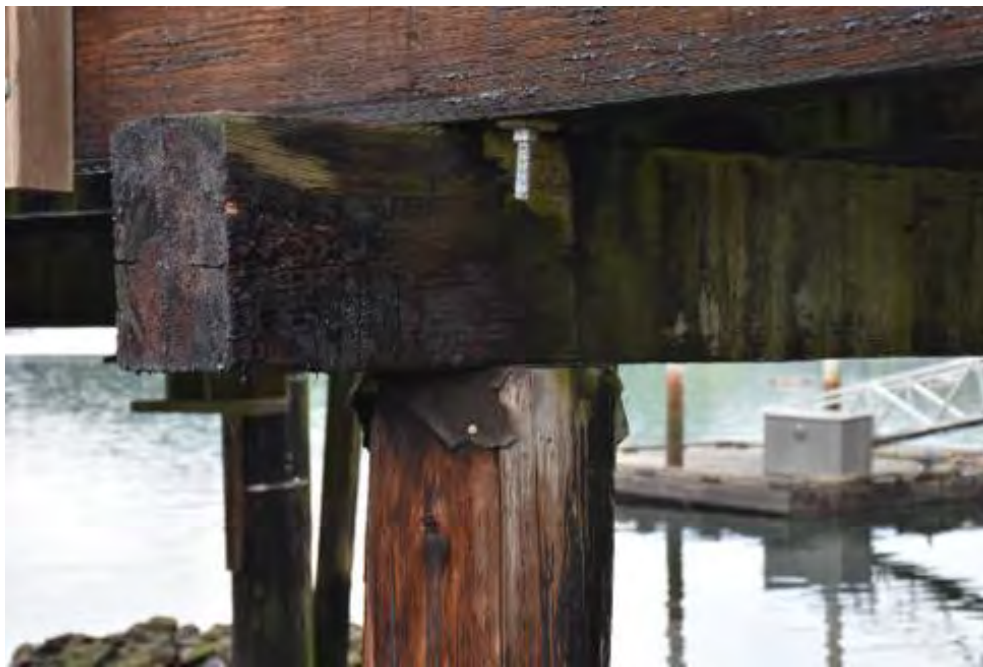
Photo 16 - Typical deteriorated capping on piles
