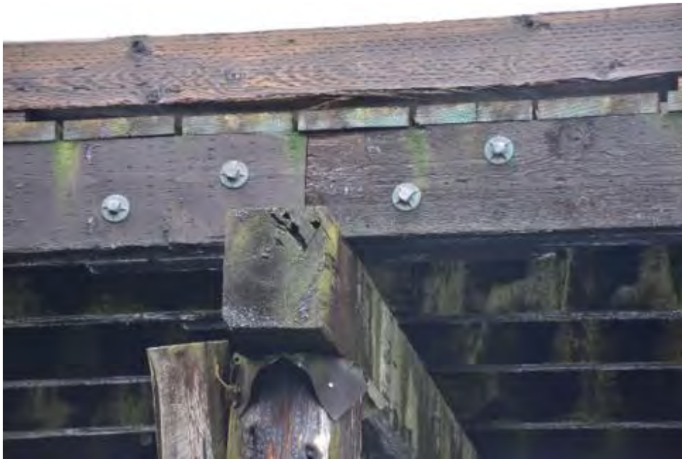
Photo 10 - Deterioration of the Pile Cap at Bent 6
