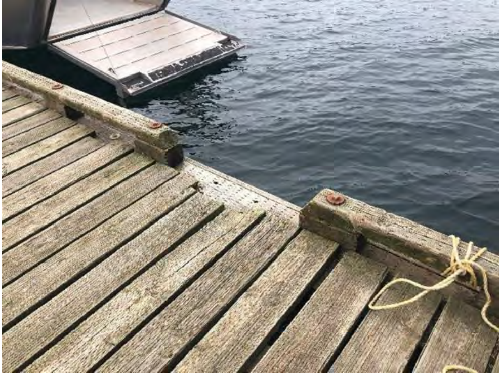
Photo 39 – Missing Bull rail on Float A
