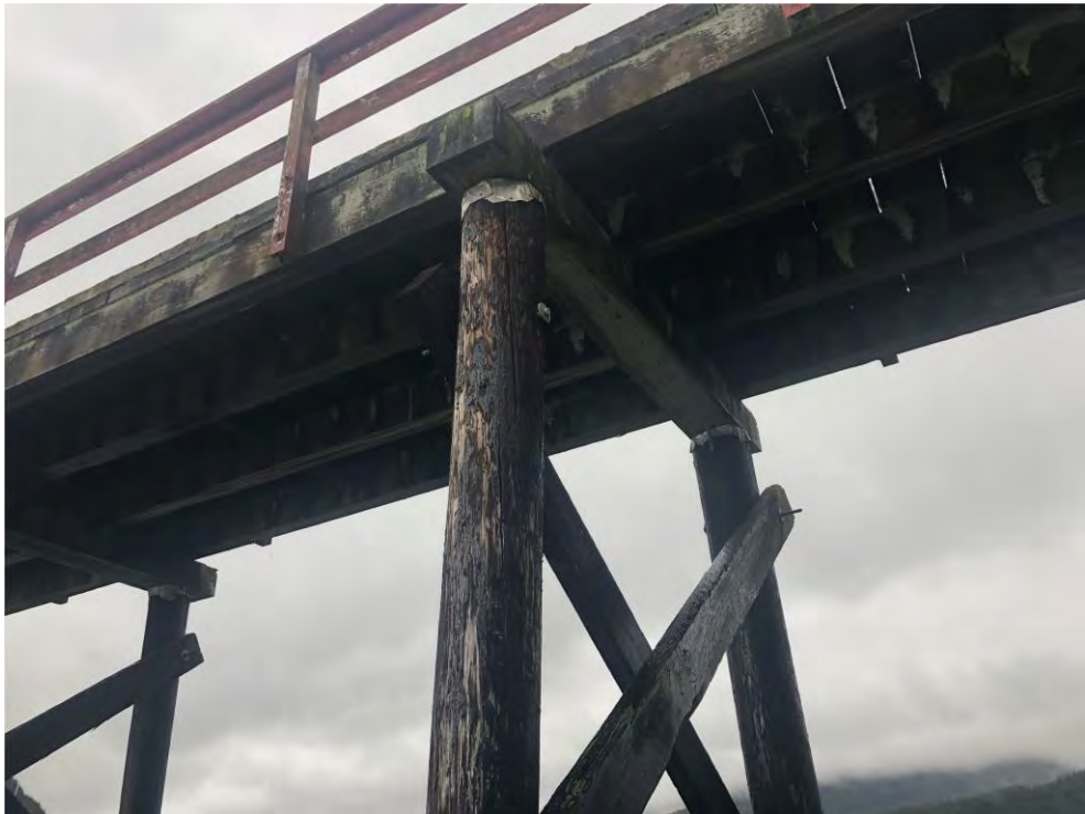
Photo 22 – Small split in Pile 10A
