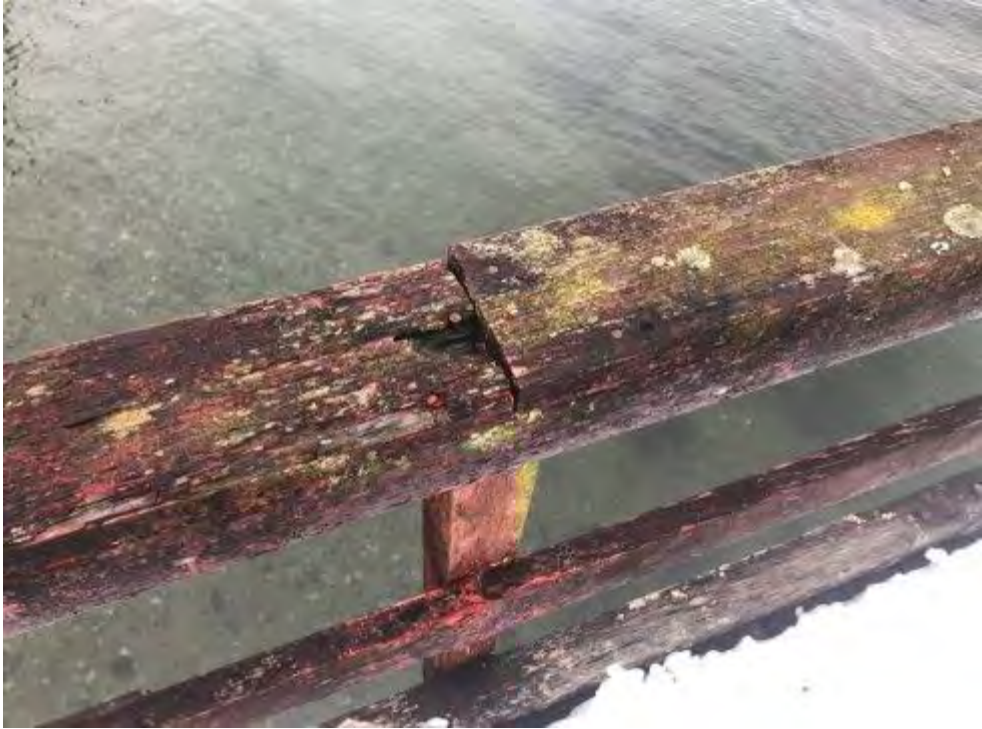
Photo 5 – Handrail deterioration between piles 7A and 8A
