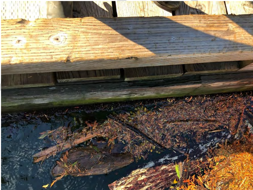
Photo 46 - Typical condition of the timber bull rails and fascia board on the Main Float
