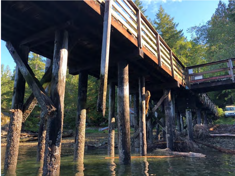
Photo 35 - Hanging side brace at pile 11B
