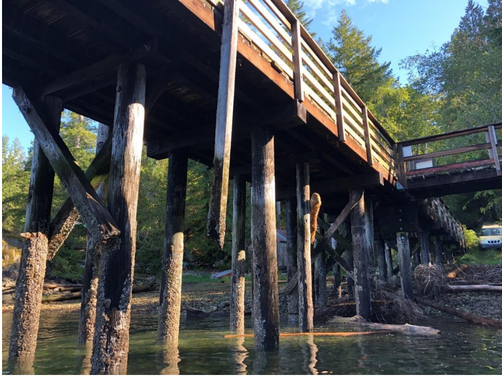
Photo 35 - Hanging side brace at pile 11B
