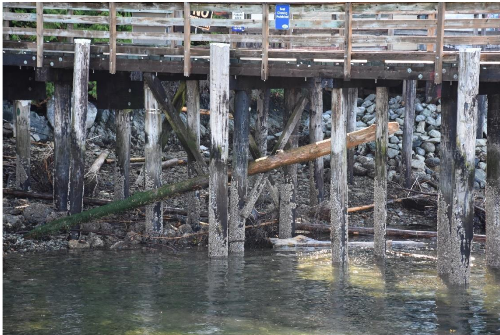
Photo 30 - North end fender piles and log debris
