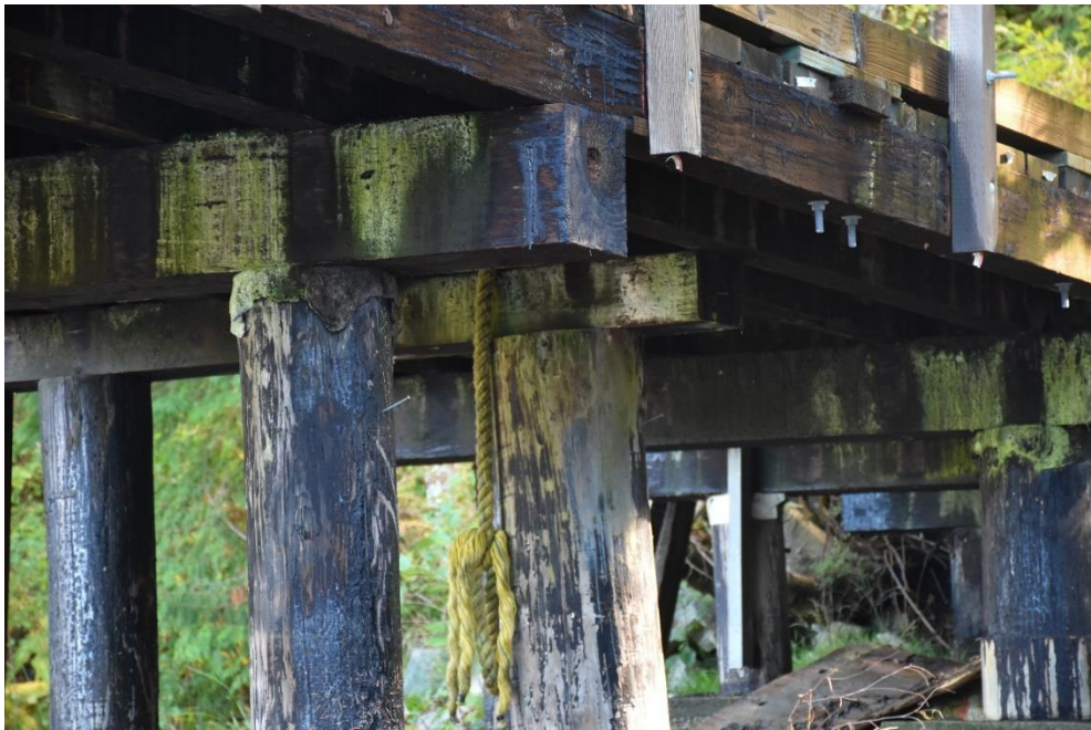
Photo 10 - Weathering and green algae growth on pile caps
