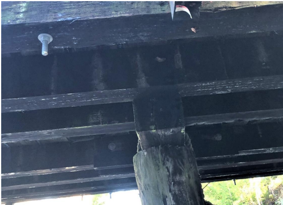
Photo 12 - Minor splitting of the pile cap at Bent 2
