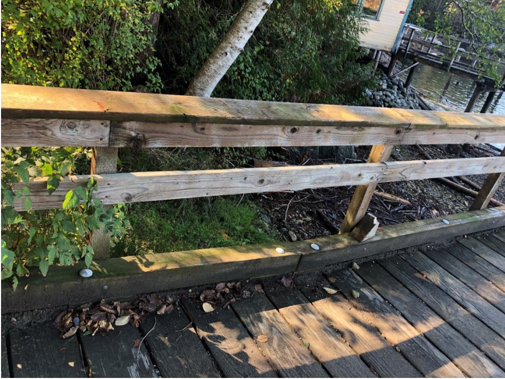
Photo 5 - Missing lower mid-rail
