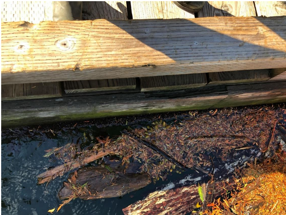
Photo 46 - Typical condition of the timber bull rails and fascia board on the Main Float
