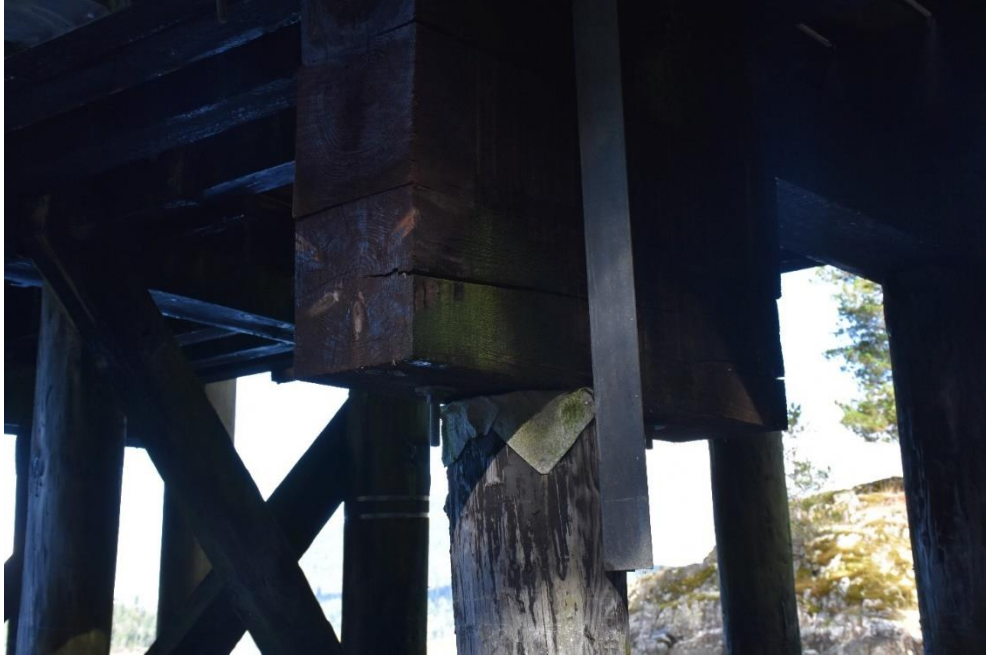
Photo 17 - Split in corbel at Bent 7
