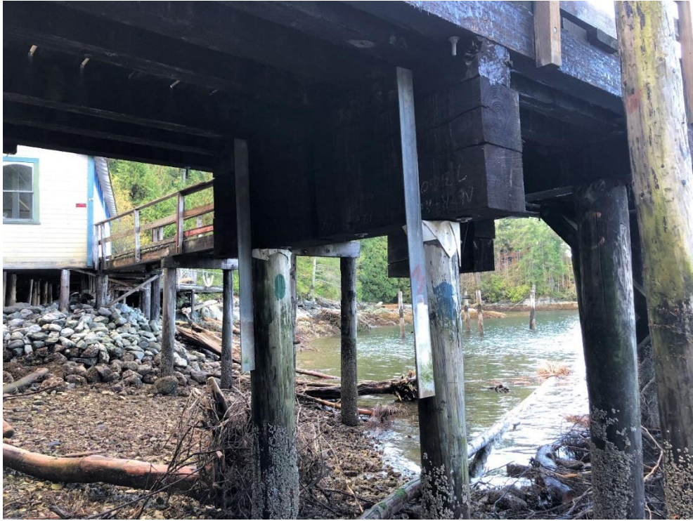
Photo 15 - Split in corbel at Bent 6
