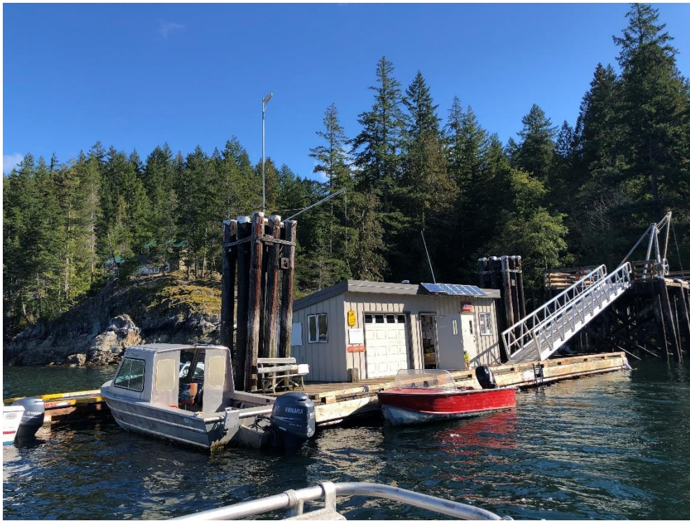
Photo 42 - General View of the Main Float
