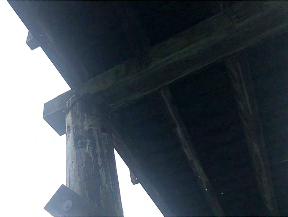
Photo 23 – Hole in Pile 12A
