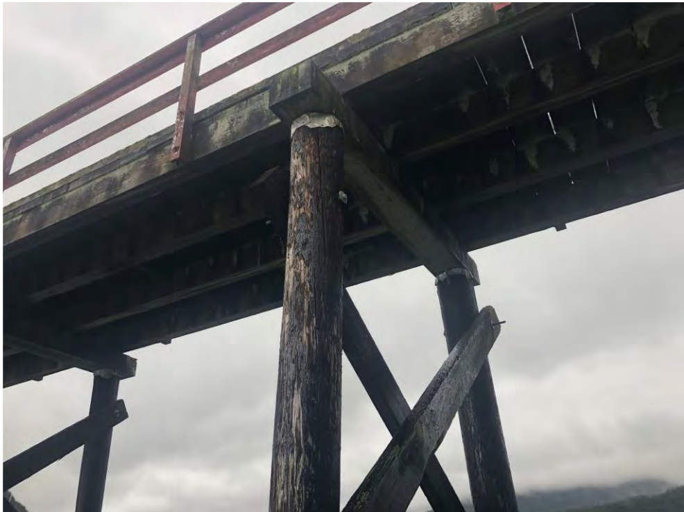
Photo 22 – Small split in Pile 10A
