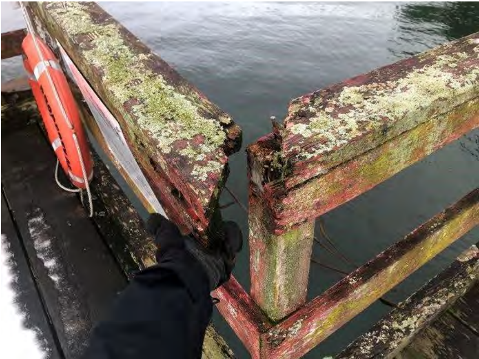
Photo 10 – Handrail deterioration between piles 14B and 14C
