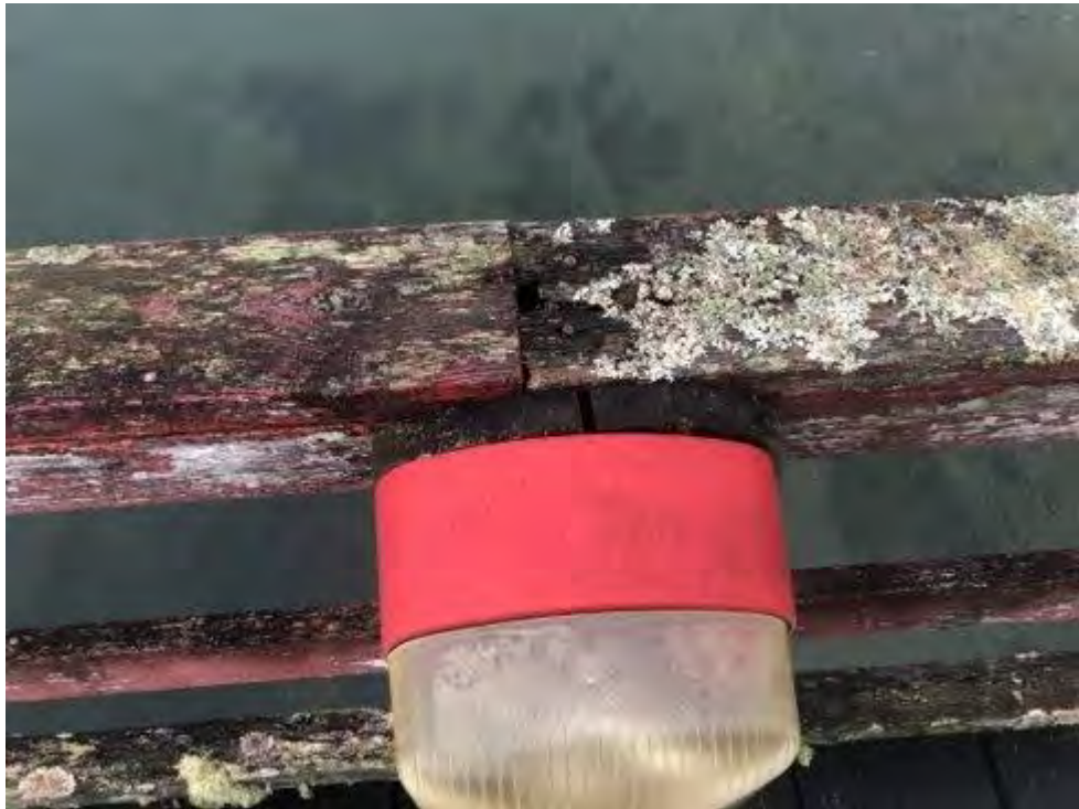
Photo 6 – Handrail deterioration between piles 8B and 9B
