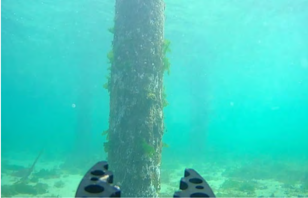
Photo 25 – Underwater image of damage to fender Pile 10B
