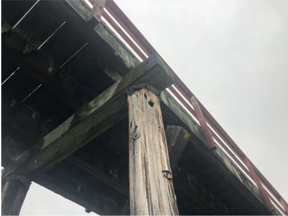
Photo 21 – Hole in Pile 9A
