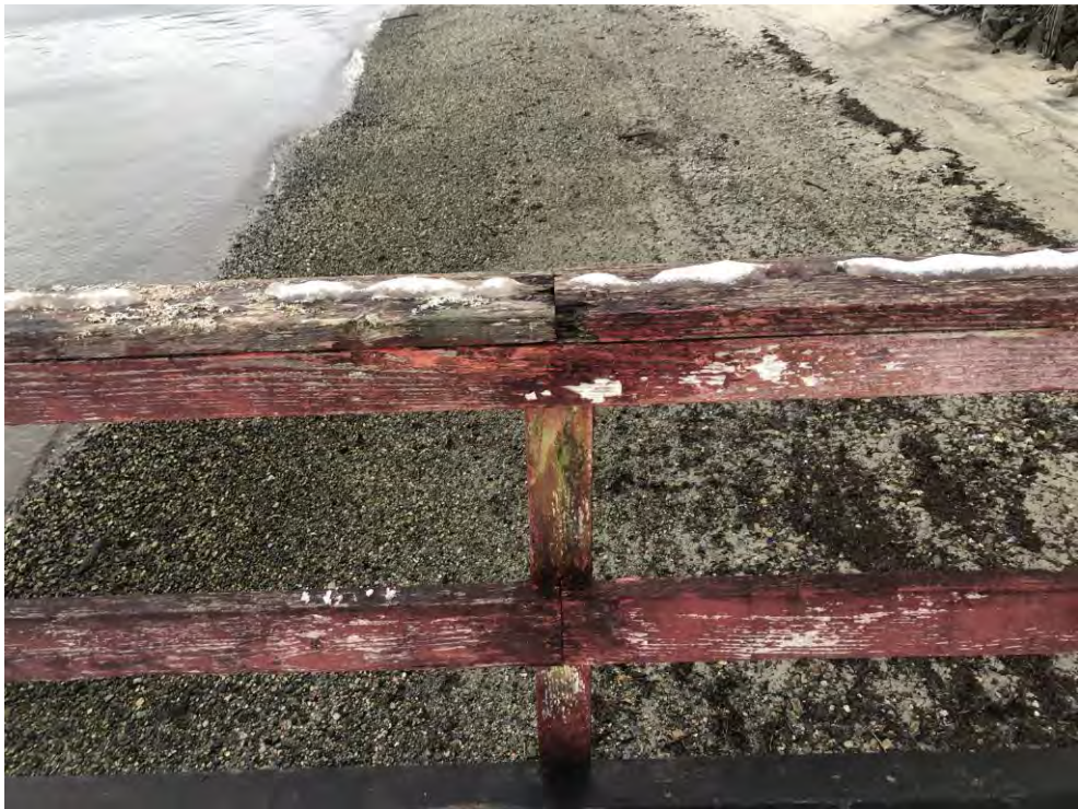
Photo 4 – Handrail deterioration between piles 4B and 5B
