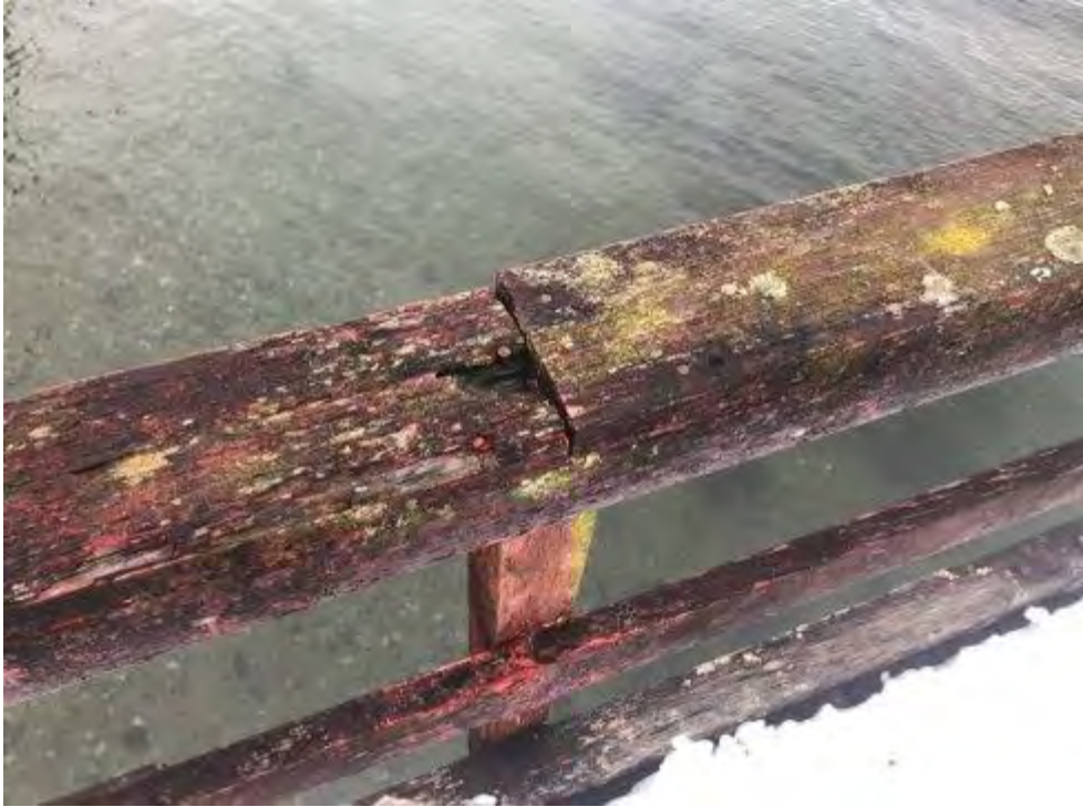
Photo 5 – Handrail deterioration between piles 7A and 8A
