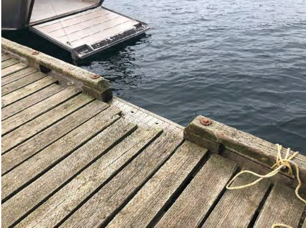
Photo 39 – Missing Bull rail on Float A
