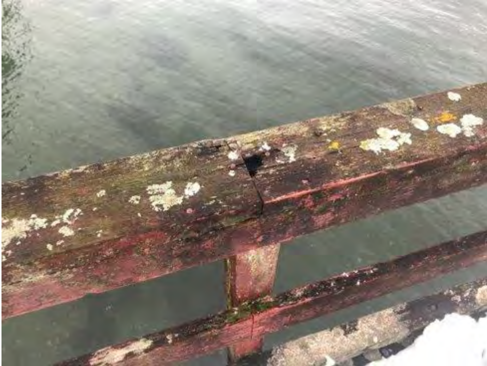
Photo 7 – Handrail deterioration between piles 9A and 10A
