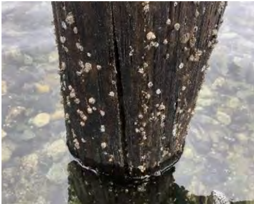
Photo 18 – Split in Pile 5A
