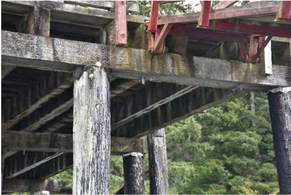
Photo 24 – Moss growth in Pile 15B
