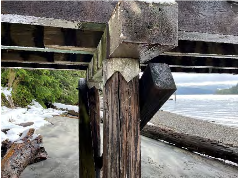
Photo 16 – Split in Pile 3B
