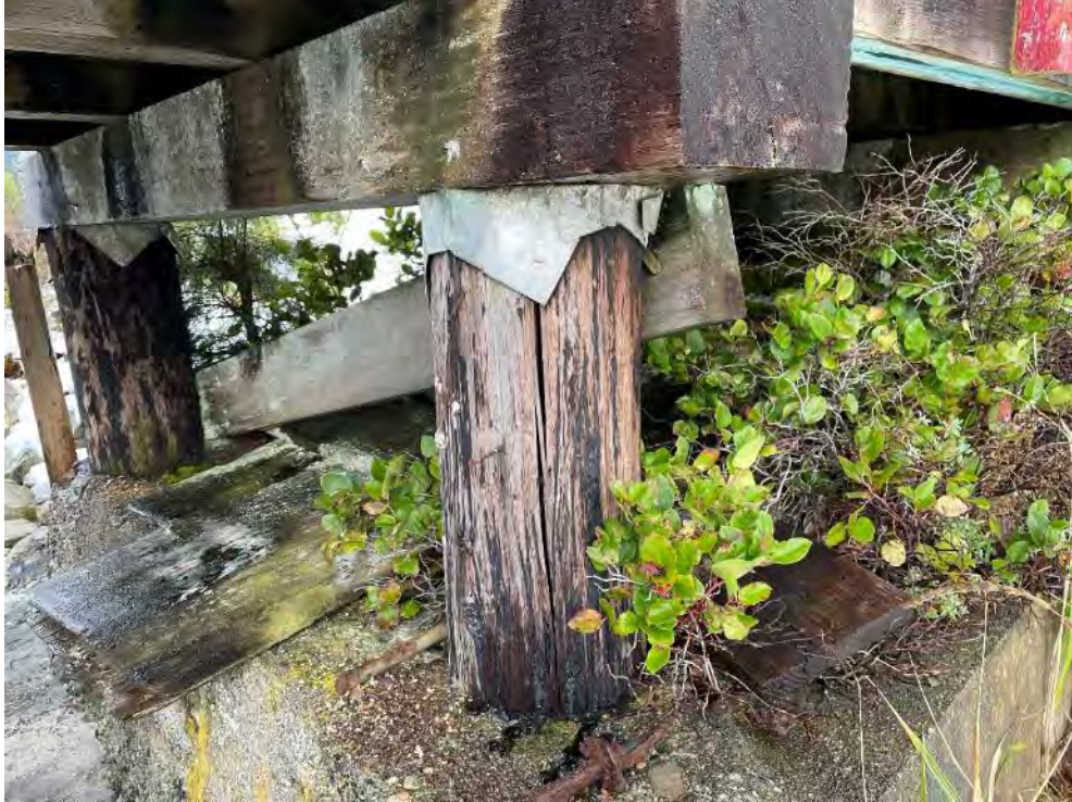
Photo 15 – Split in Pile 2A
