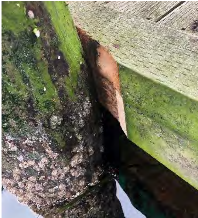
Photo 42 – Wearing to Float A from South Mooring Piles
