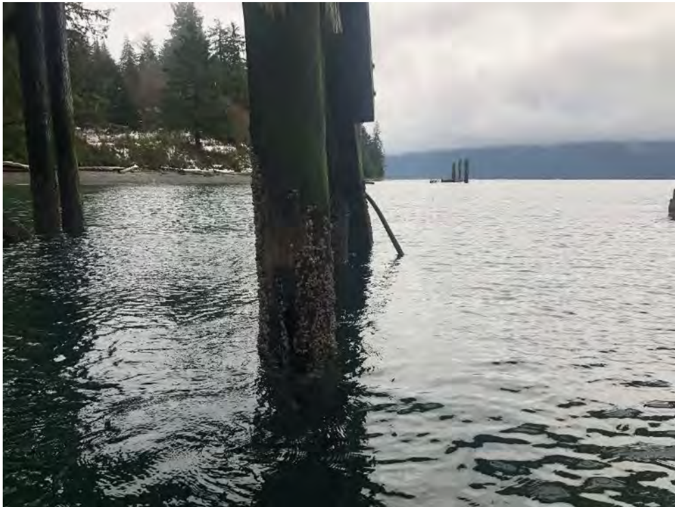
Photo 28 – Fender Pile 15C
