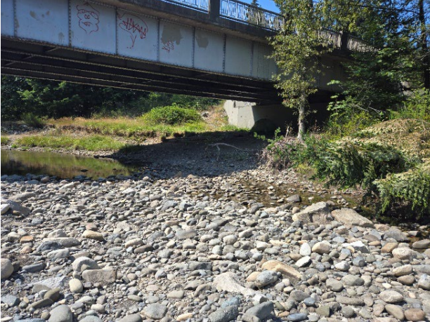
Photo 13: No Bank Armouring and Some Erosion Evident on the Left Abutment of the Hwy 19a Bridge (August 7, 2024)
