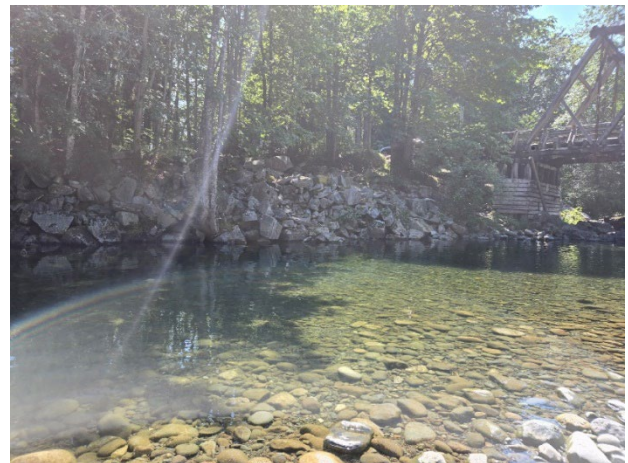
Photo 12: Steep and Varied Riprap Showing Some Material Loss on the Right Abutment of the Regent Road Bridge (August 7, 2024)
