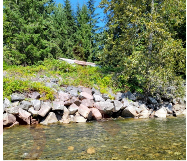
Photo 2: Some Minor Riprap Loss at the Toe of Slope Upstream of Hwy 19a Bridge (August 7, 2024)
