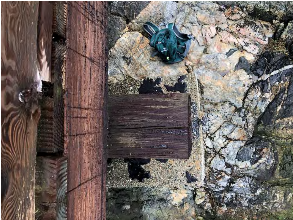
Photo 8 - Minor splitting of the Pile cap at Bent 4
