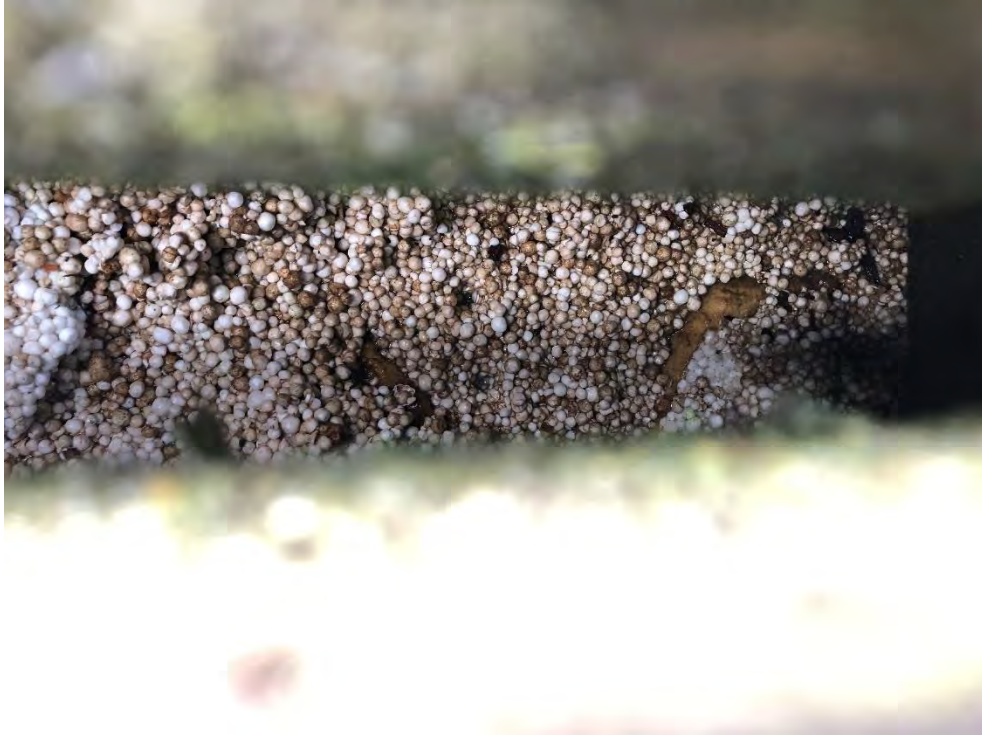
Photo 33 - Condition of exposed uncoated styrofoam billets
