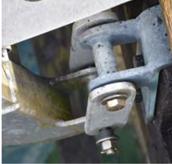
Photo 23 - Gangway Upper Hinge Connection with loose bolt
