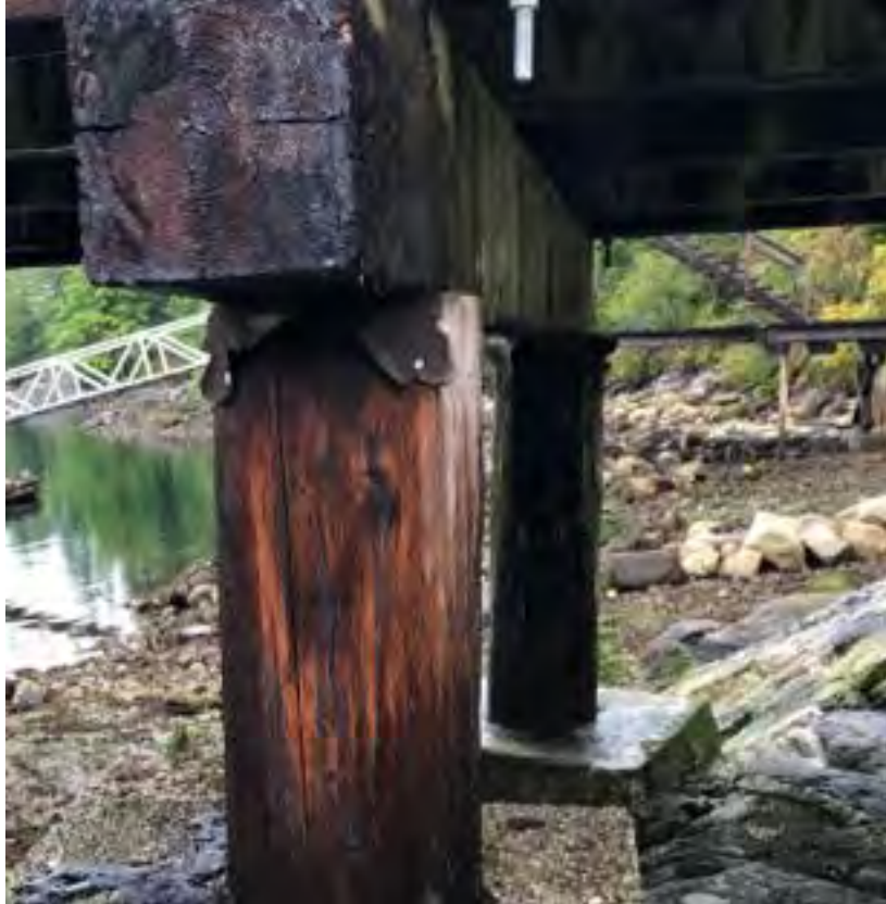
Photo 17 - Minor splitting on Pile 4B
