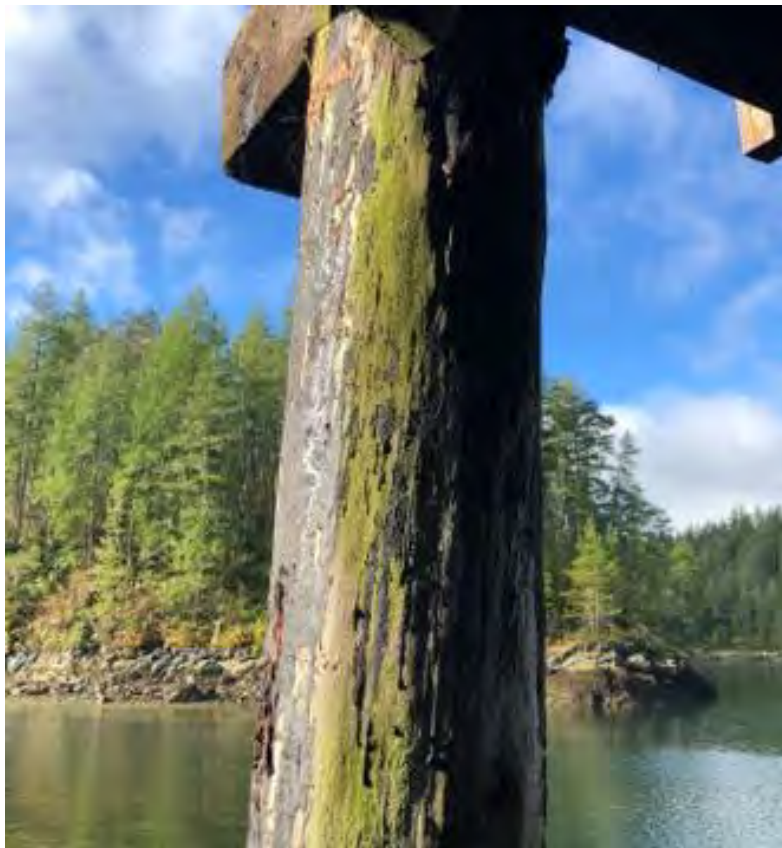
Photo 14 - Typical weathering and green algae growth on piles
