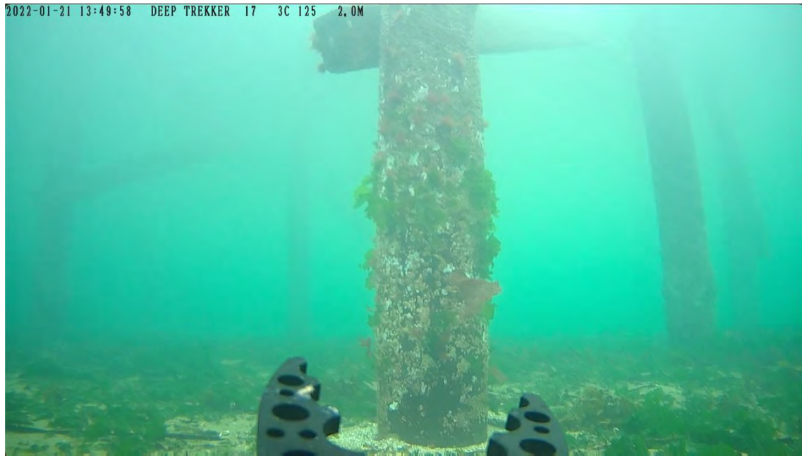
Photo 15 - Typical condition of underwater piles
