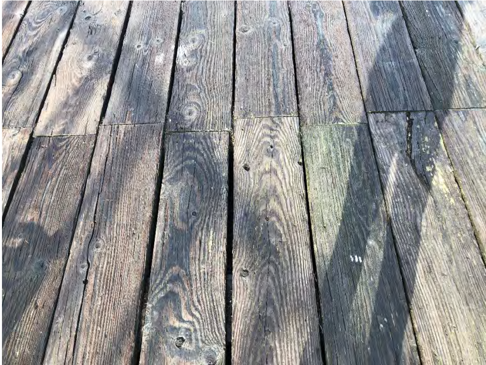
Photo 25 - Typical condition of the timber decking
