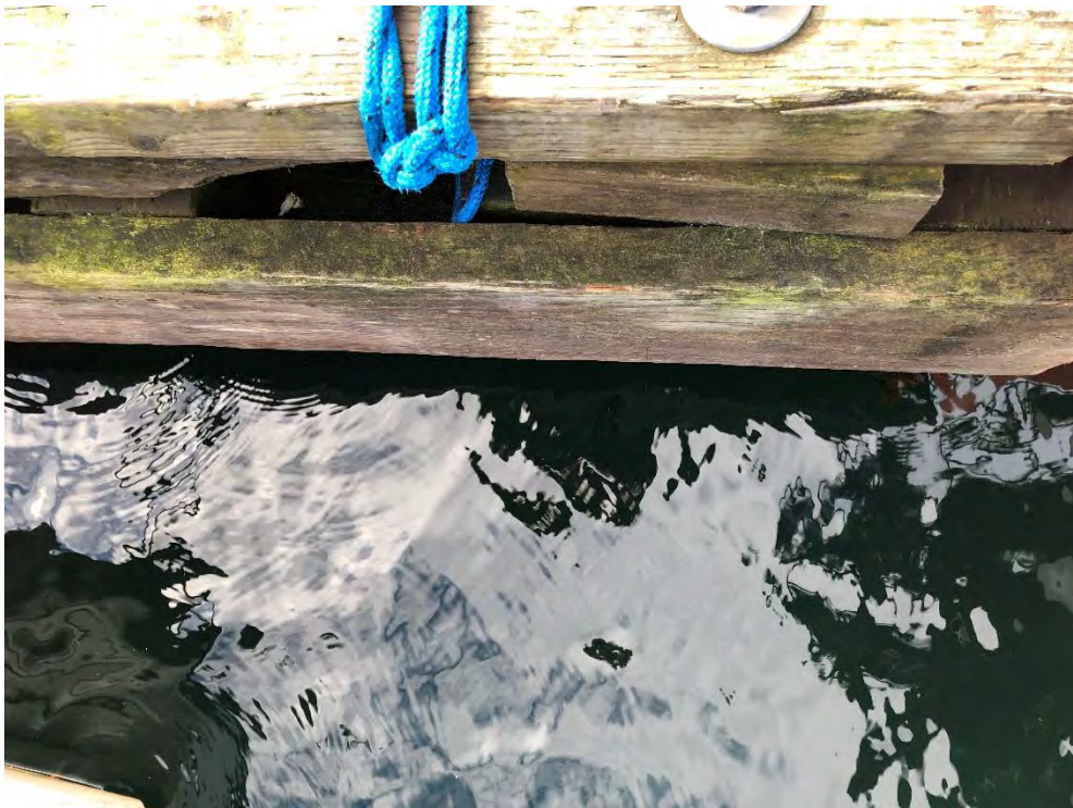
Photo 26 - Typical condition of the timber bull rails and fascia board
