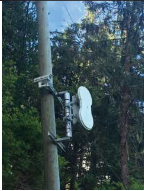
2. Point to point radio transceiver at Walters Lodge on Walter Island
