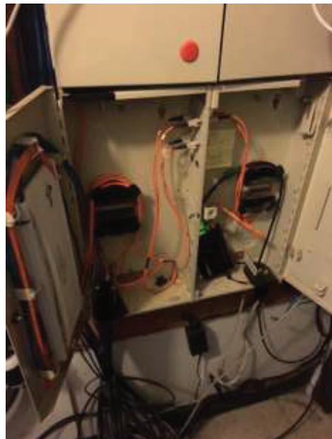
Fibre Entrance Panel within school building
