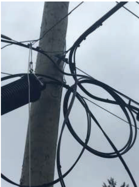
Presents of Telus fibre on Walters Island directly adjacent to the TELUS microwave site
