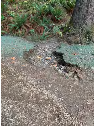
Photo 3: Sta. 0+200 (LHS) Erosion
