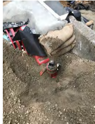
Photo 4: Gate Valve Grease Nipples
