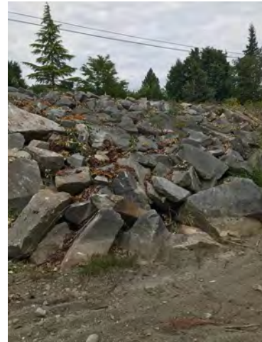
Photo 4: Voids and Instability in Riprap, E Section
