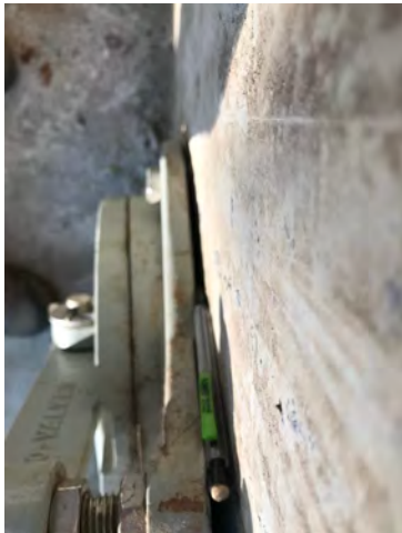
Photo 1: Re-Installed Flap Gate not Mounted Flush
