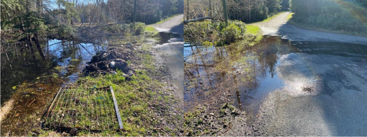
Figure 38 and Figure 39. The grate that was covering the culvert has been removed, the culvert is not completely blocked and causing water to flow over the road. March 26, 2024.
