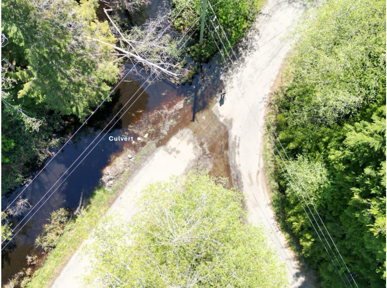
Figure 56. Aerial photo of Kw'as Bay Road flooding due to the blocked, beaver dammed, culvert. May 1, 2024.
