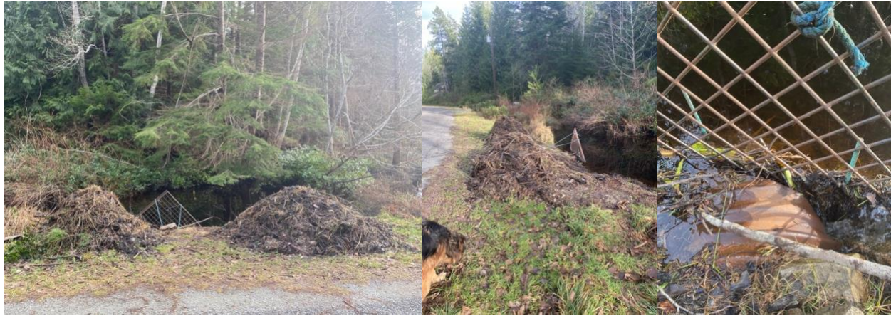
Figure 35, Figure 36, Figure 37. The culvert is completely blocked by a beaver dam built on the grate placed in front of the culvert. The grate in front of the culvert provides the beaver with a solid and convenient place to build a dam. Notice the piles of organic soils and debris that are piled on the edge of the road from the last time the beaver dam was removed. January 12, 2021.
