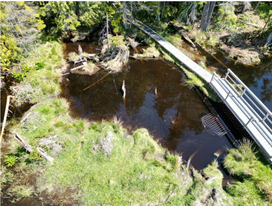
Figure 51. Aerial photo, close up of existing pond leveler, notice the rust on the intake cage, which is placed too close to the beaver dam. May 1, 2024.
