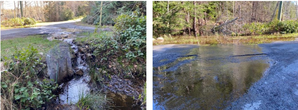
Figure 40 and Figure 41. The road surface is eroding due to consistent water flow over the road. March 26, 2024.
