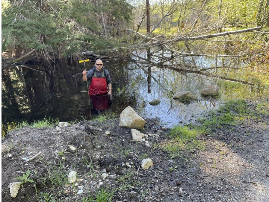
Figure 42. Chris Holtslag is standing at the inlet of the culvert which is totally submerged and blocked. A culvert protection fence is proposed for this location to reduce the risk of road failure and ecological impacts from continually unblocking the culvert. May 1, 2024.
