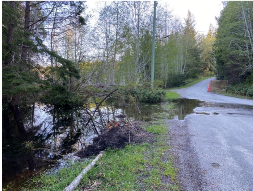
Figure 33. The culvert at Kw'as bay road is completely blocked by a beaver dam and water is flowing over the road. Notice the pile of organic soil and debris placed on the side of the road, from the last time the culvert was unblocked. May 2, 2022.
