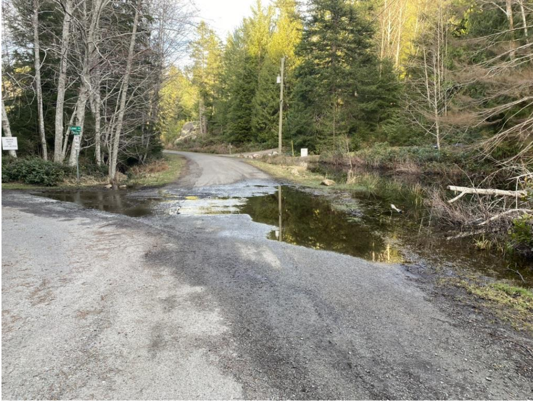
Figure 45. The road culvert has been completely blocked for over a year, water is flowing over the road. March 6, 2025.
