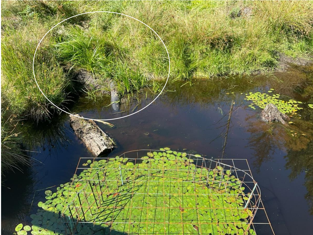
Figure 17. The intake cage for the pond leveler was built with inappropriate materials, which are starting to rust. Additionally, this cage was placed too close to the dam where sediment will accumulate. This photo was taken during low water conditions, mid August, and demonstrates that the wetland pool upstream of the dam would not be de-watered during construction. Note the pond leveller is exposed. This pond leveller would be replaced as part of the project, using the same outlet elevation, therefore the pool wetland would not be dewatered. August 29, 2024.
