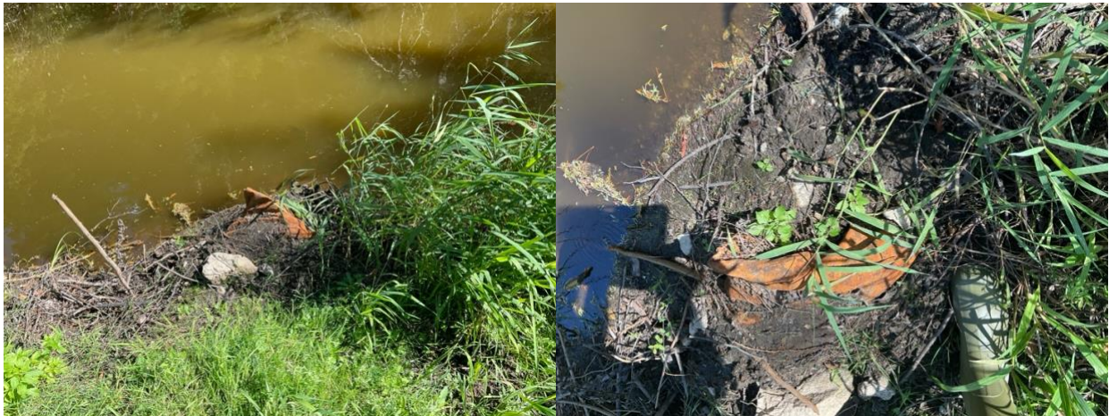
Figure 43 and Figure 44. Now that water levels have dropped in the dry time of year, the culvert is exposed. The inlet of the culvert is damaged and bent out of shape from attempts to use a log with a backhoe to dislodge the beaver dam. August 29, 2024.
