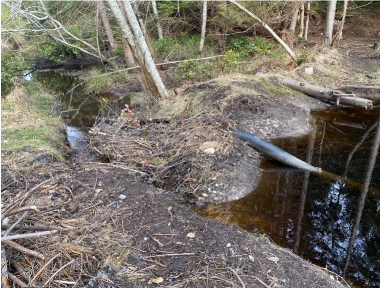
Figure 22. Left. This beaver dam had a pond leveler installed that is not functioning as intended. The pipe is too small diameter, and the intake not properly placed. The beaver dam still needed to be breached to manage water levels. March 13, 2023.
