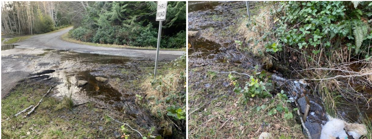
Figure 46. Left. Water flowing over Kw'as Bay Rd is eroding the road surface. March 6, 2025.
