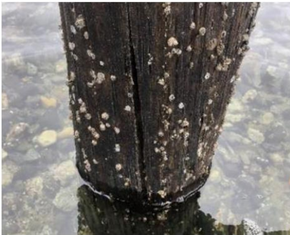
Photo 18 – Split in Pile 5A
