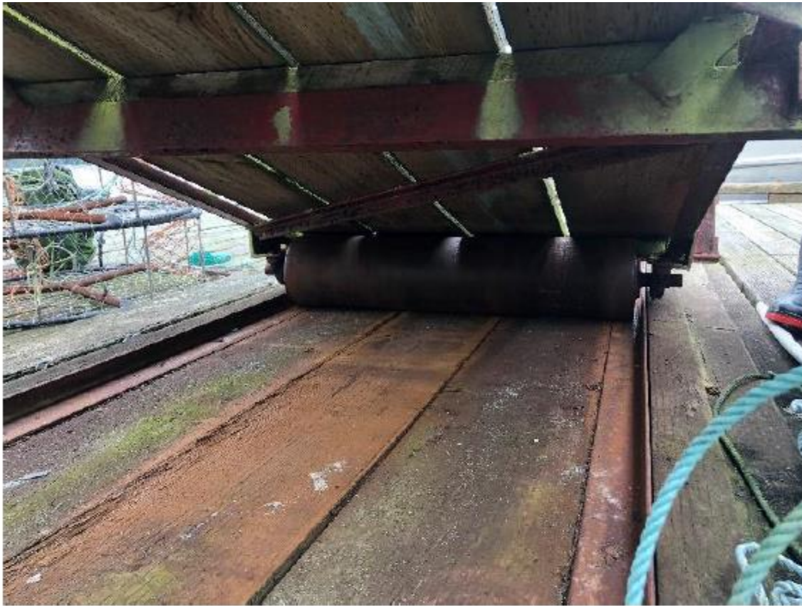
Photo 33 – Gangway Timber Slider Plate and Roller
