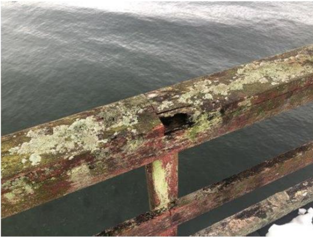
Photo 9 – Handrail deterioration between piles 12A and 13A
