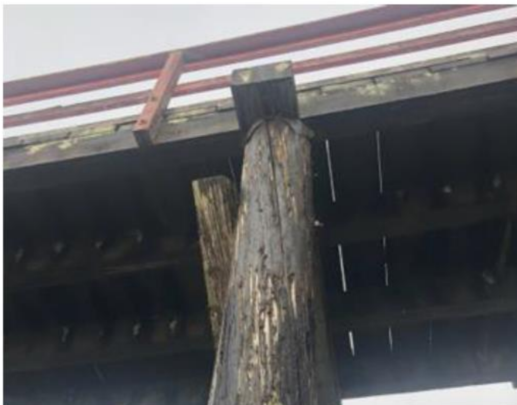
Photo 20 – Split in Pile 8A
