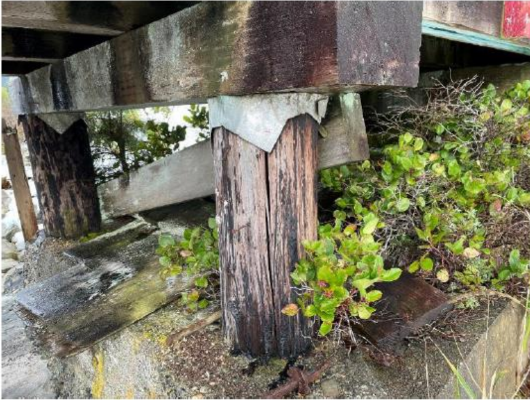
Photo 15 – Split in Pile 2A
