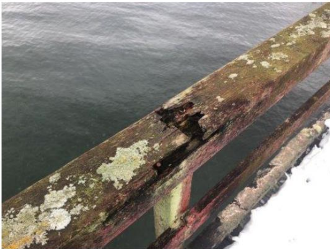
Photo 8 – Handrail deterioration between piles 11A and 12A
