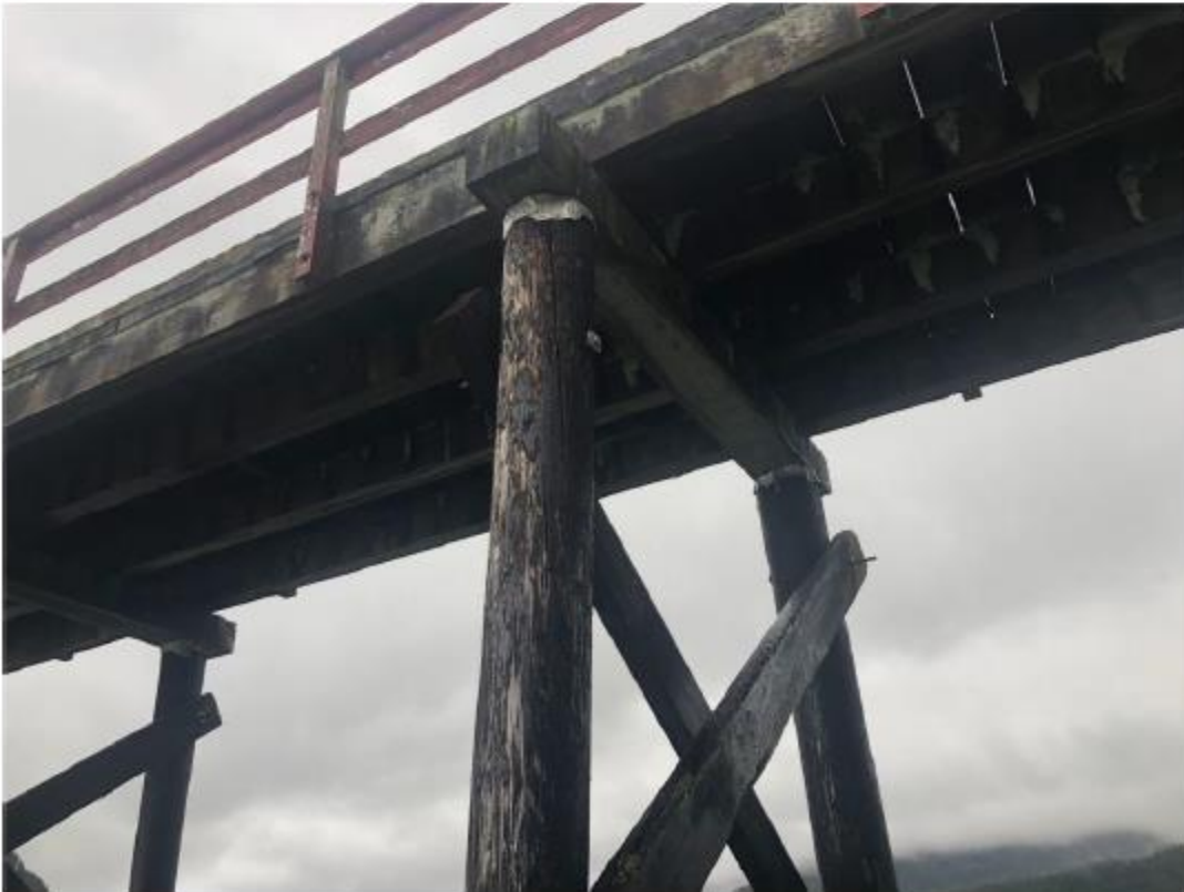
Photo 22 – Small split in Pile 10A
