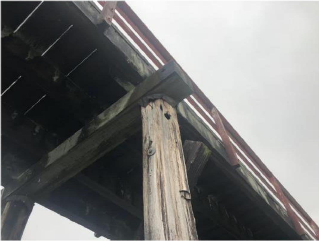
Photo 21 – Hole in Pile 9A
