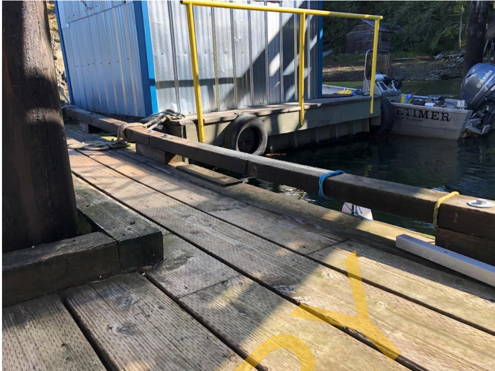
Photo 47 - Flotation loss at centre of the Main Float on the east end
