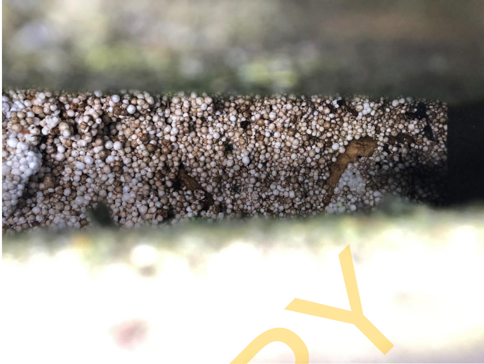
Photo 33 - Condition of exposed uncoated styrofoam billets
