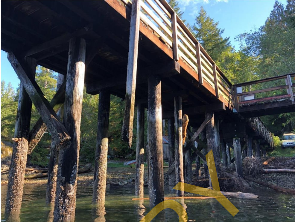
Photo 35 - Hanging side brace at pile 11B
