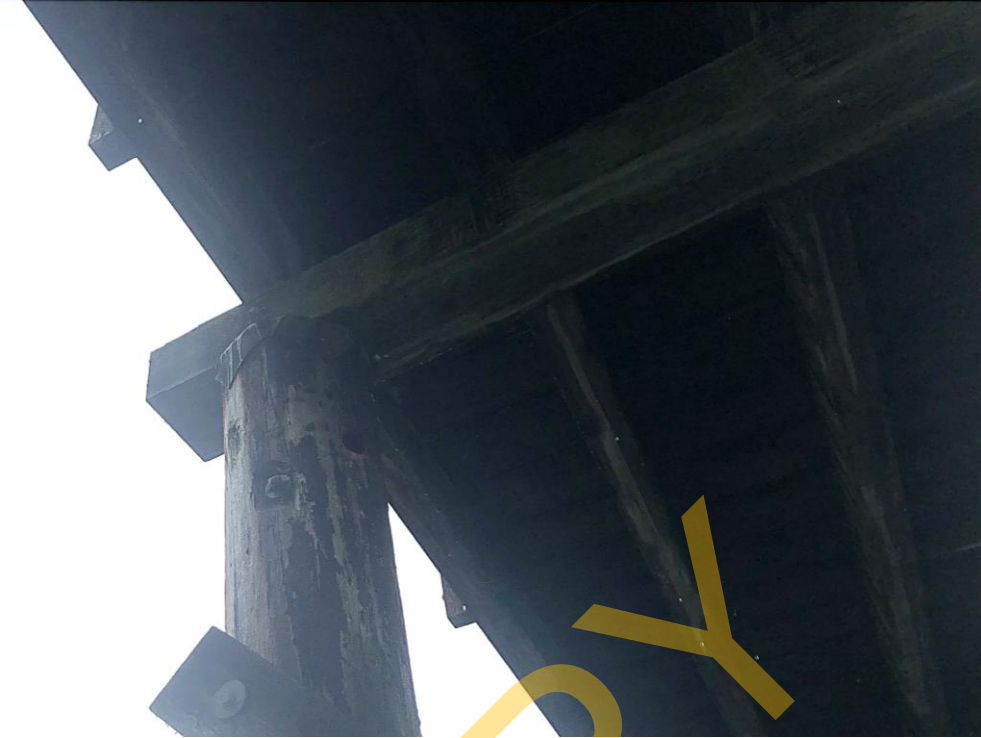
Photo 23 – Hole in Pile 12A
