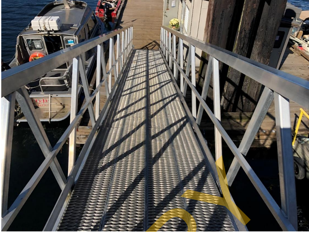
Photo 39 - General View of Aluminum Gangway
