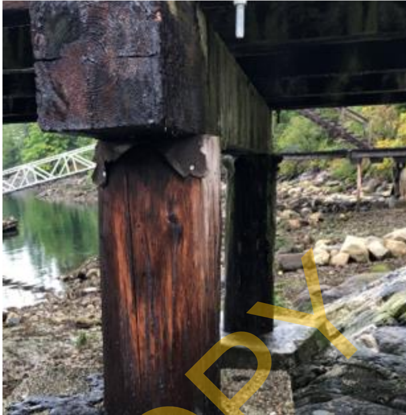
Photo 17 - Minor splitting on Pile 4B
