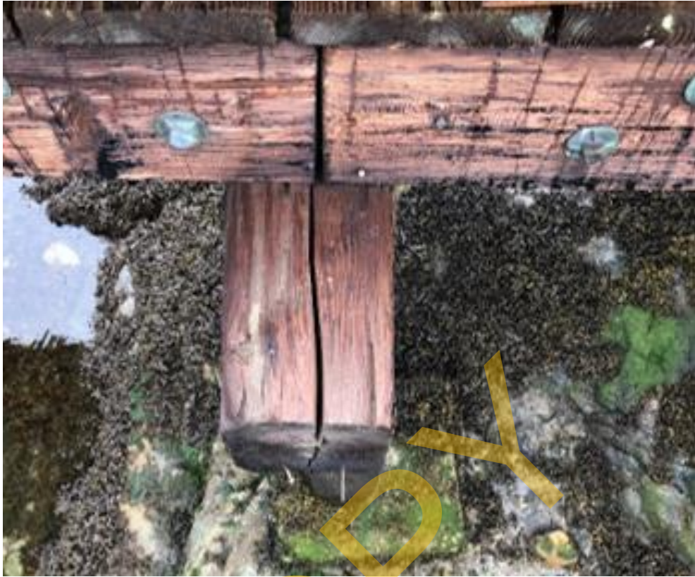
Photo 9 - Severe splitting of the Pile cap at Bent 5
