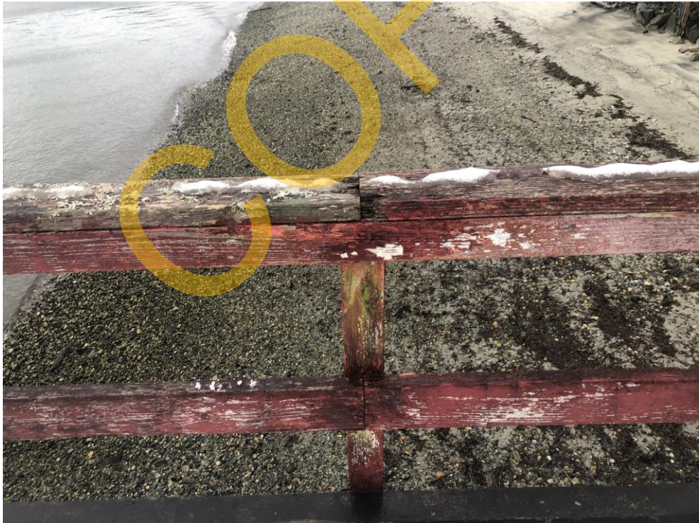
Photo 4 – Handrail deterioration between piles 4B and 5B
