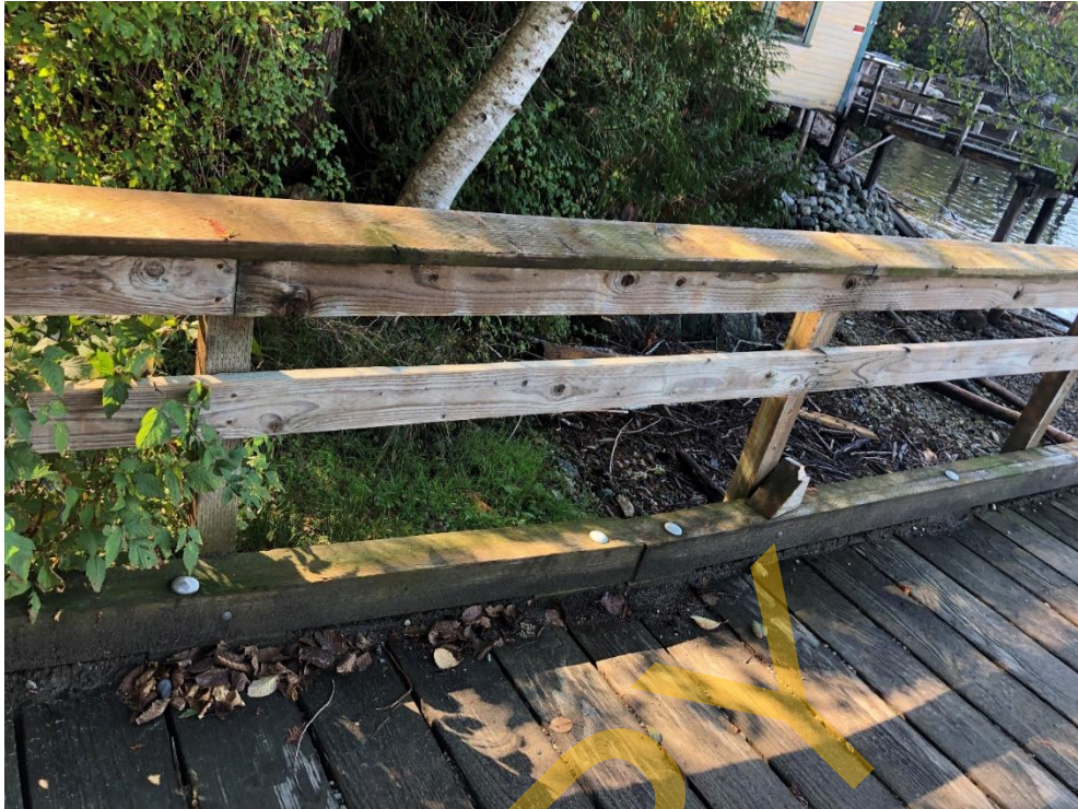
Photo 5 - Missing lower mid-rail
