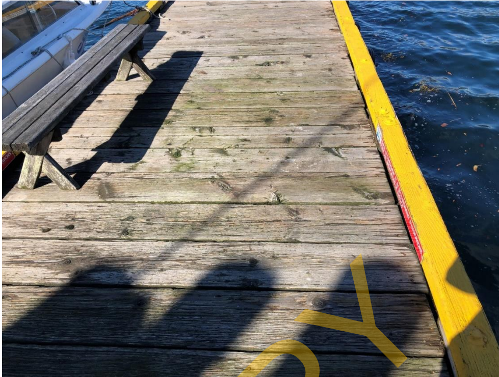
Photo 59 - Typical condition of the Seaplane Float deck
