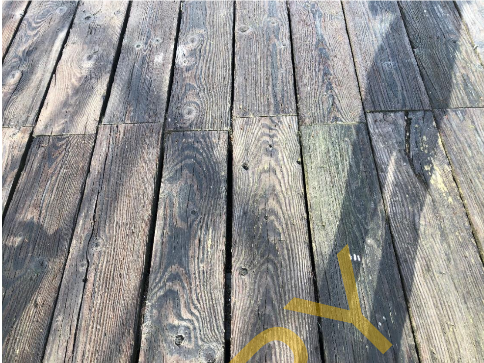
Photo 25 - Typical condition of the timber decking
