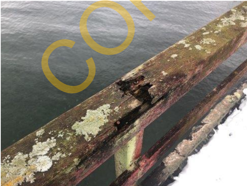
Photo 8 – Handrail deterioration between piles 11A and 12A
