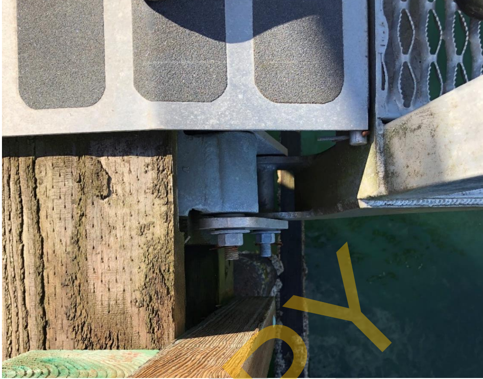
Photo 41 - Gangway Upper Hinge Connection
