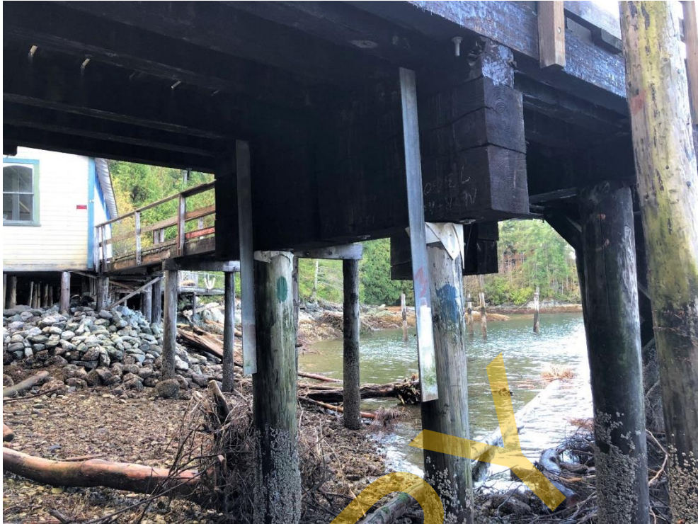
Photo 15 - Split in corbel at Bent 6
