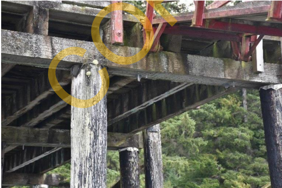
Photo 24 – Moss growth in Pile 15B
