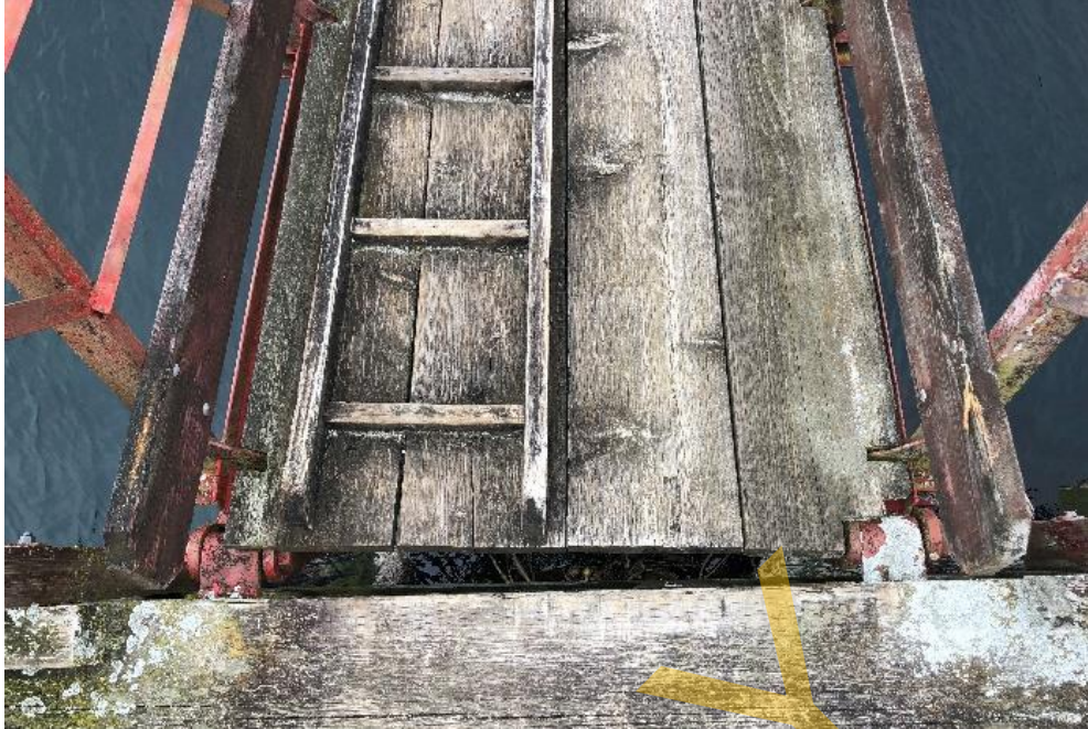
Photo 31 – Gangway Upper Hinge Connection
