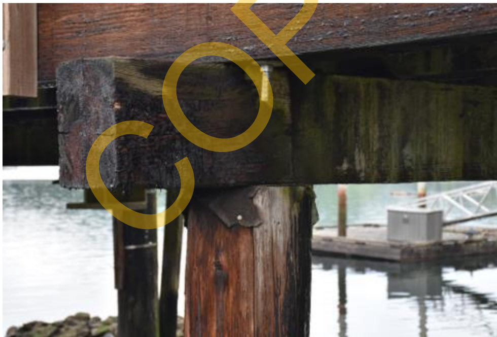
Photo 16 - Typical deteriorated capping on piles
