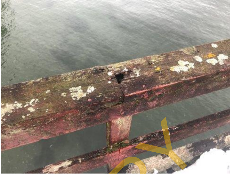
Photo 7 – Handrail deterioration between piles 9A and 10A
