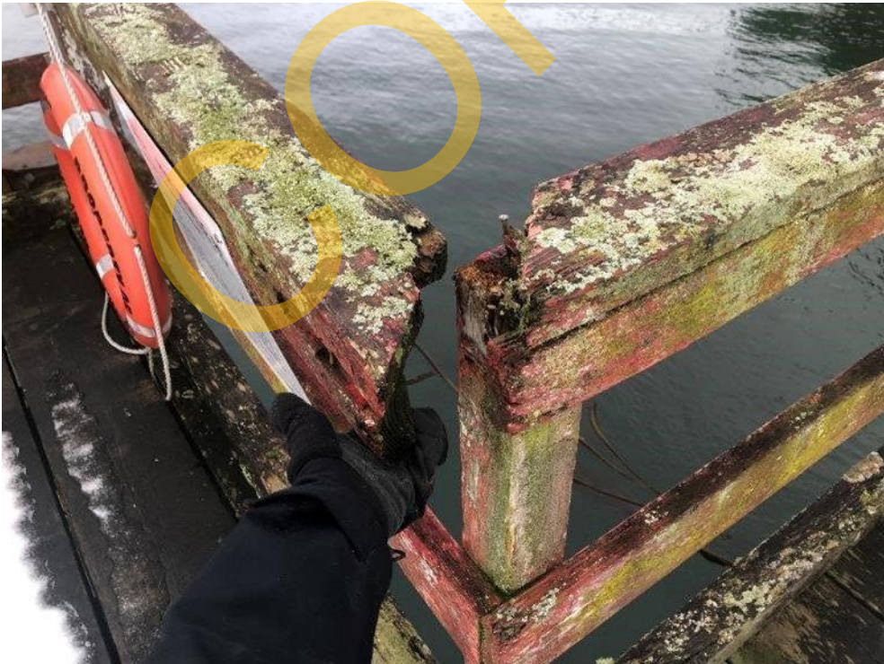
Photo 10 – Handrail deterioration between piles 14B and 14C
