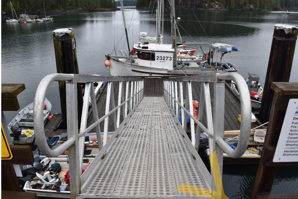
Photo 21 - General View of Aluminum Gangway
