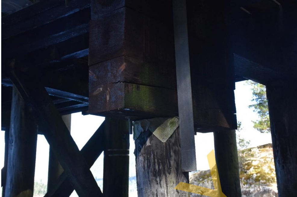
Photo 17 - Split in corbel at Bent 7
