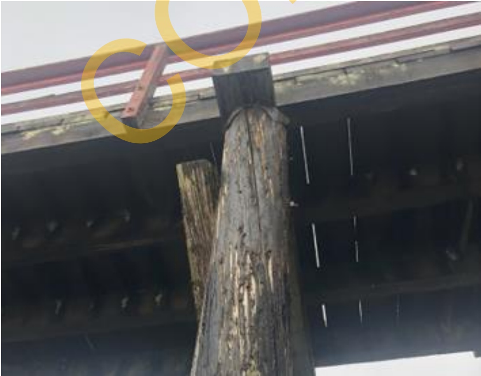
Photo 20 – Split in Pile 8A
