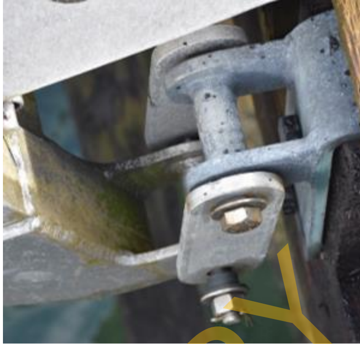
Photo 23 - Gangway Upper Hinge Connection with loose bolt
