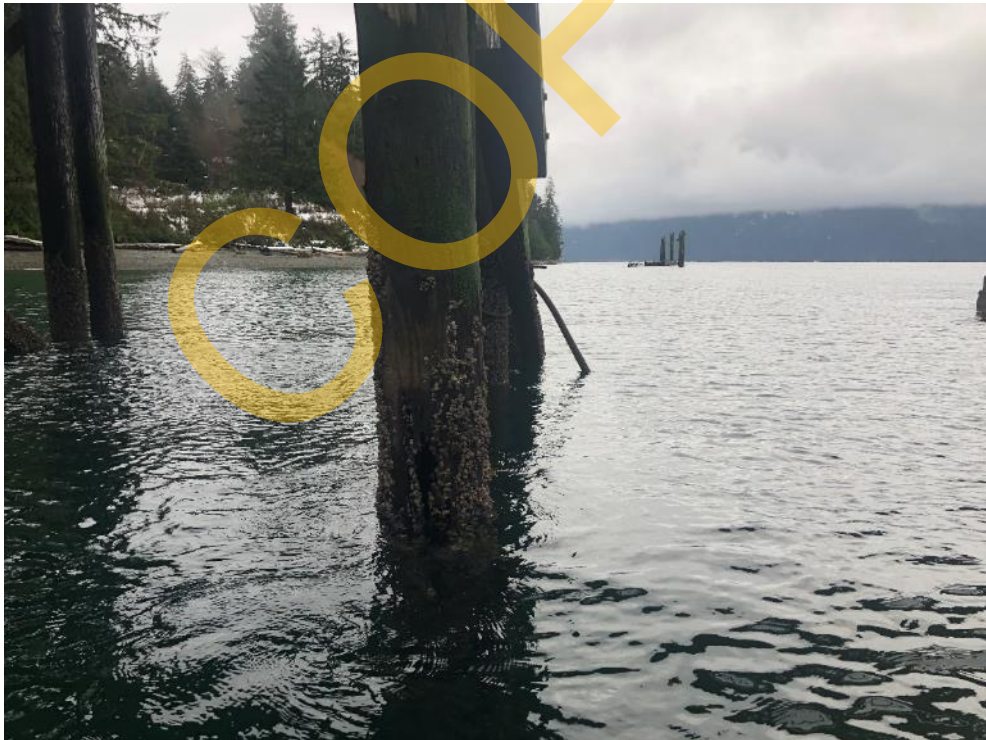
Photo 28 – Fender Pile 15C
