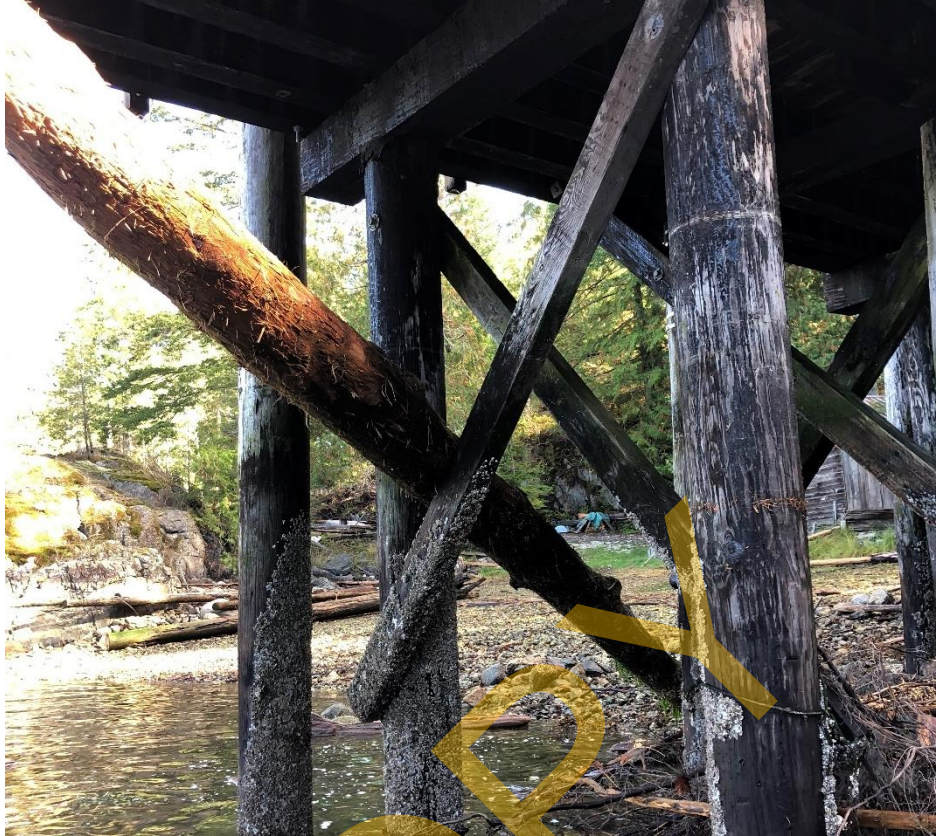
Photo 33 - Log resting on the Cross Bracing
