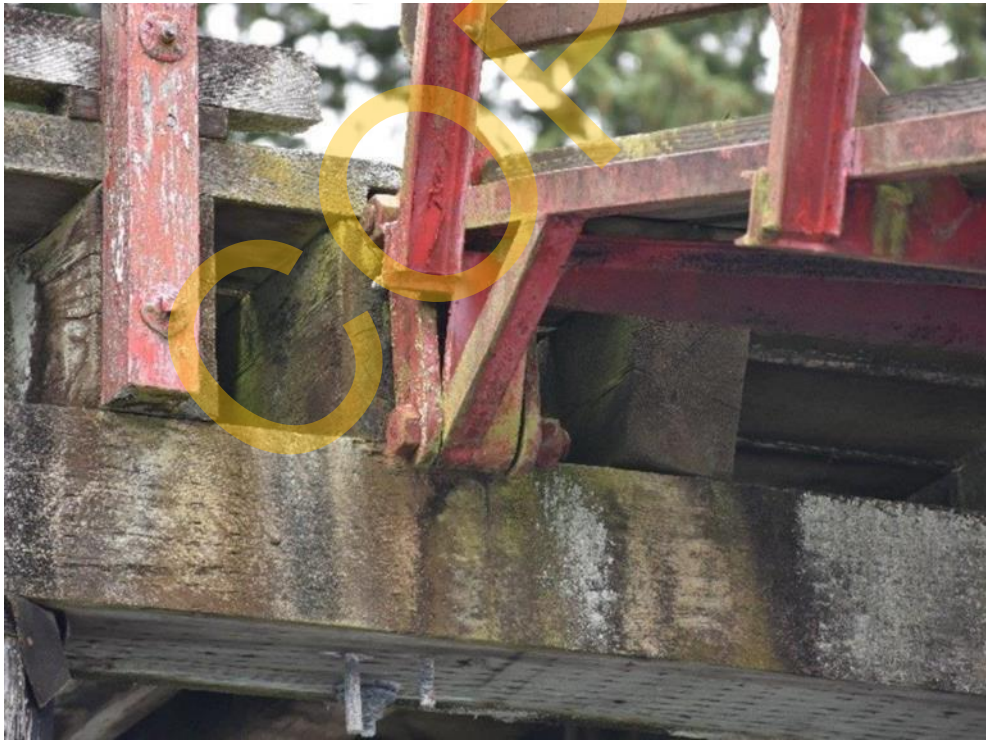
Photo 32 – Gangway Upper Hinge Connection
