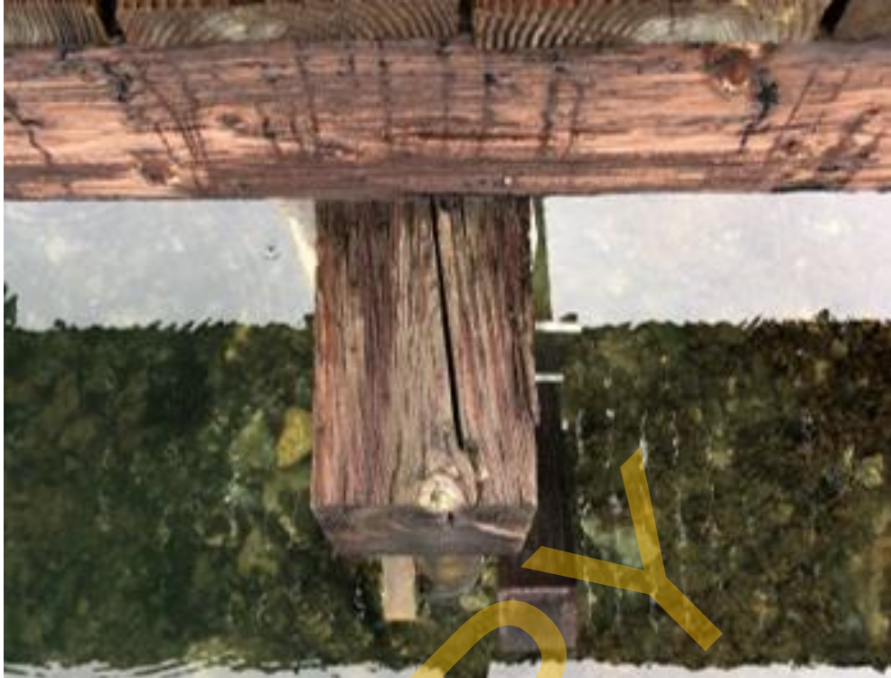
Photo 11 - Moderate to Severe splitting of the Pile cap at Bent 6
