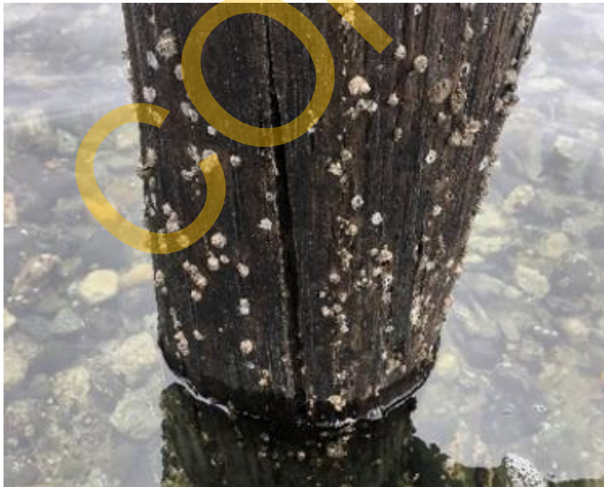
Photo 18 – Split in Pile 5A
