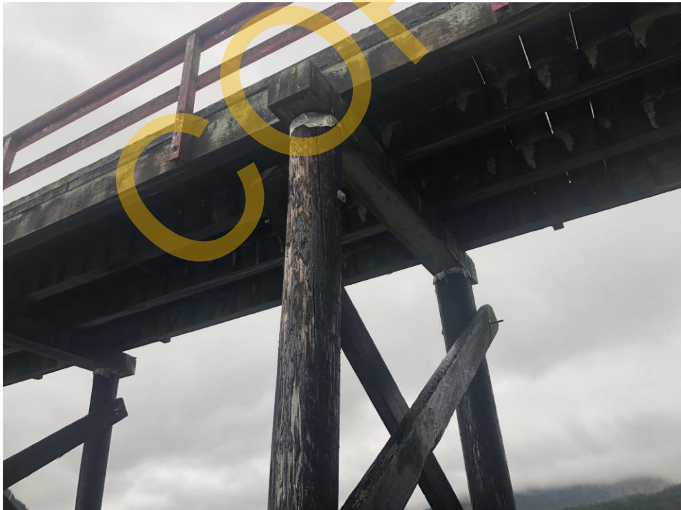
Photo 22 – Small split in Pile 10A
