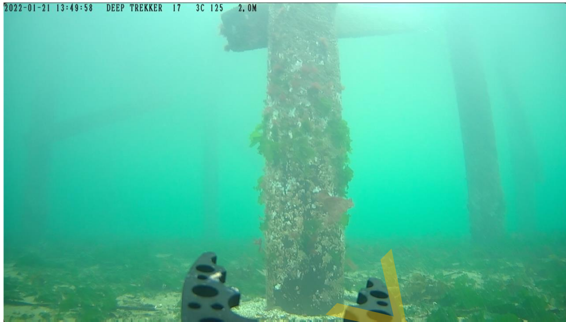
Photo 15 - Typical condition of underwater piles
