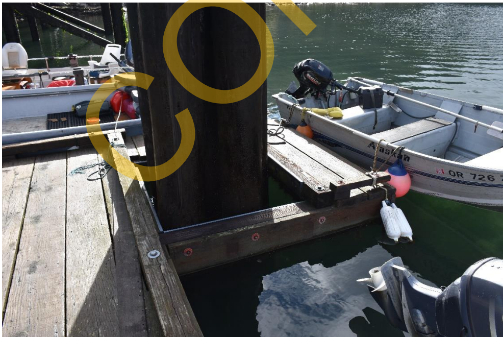
Photo 34 - South Mooring Well with significant flotation loss
