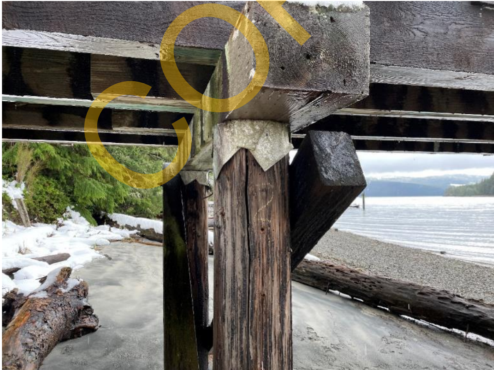
Photo 16 – Split in Pile 3B
