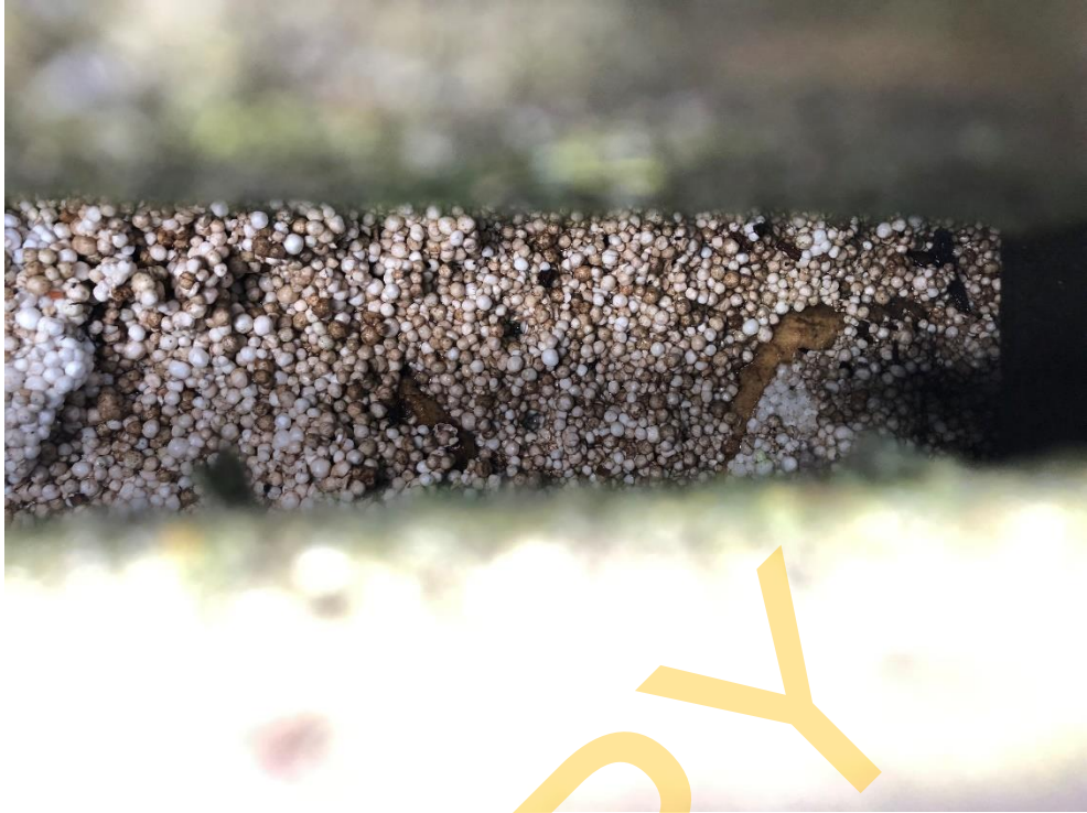
Photo 33 - Condition of exposed uncoated styrofoam billets
