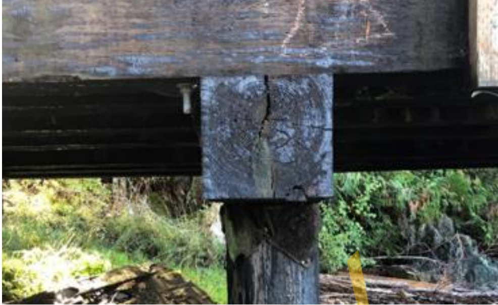
Photo 11 - Split at the north end of the pile cap at Bent 1
