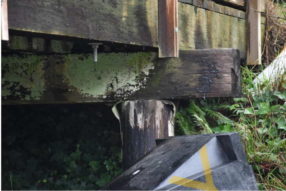
Photo 7 - Weathering and green algae growth on Pile Caps
