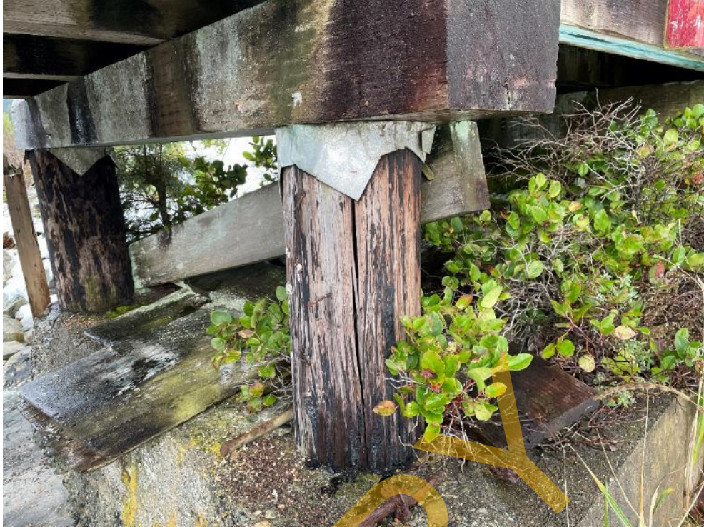
Photo 15 – Split in Pile 2A
