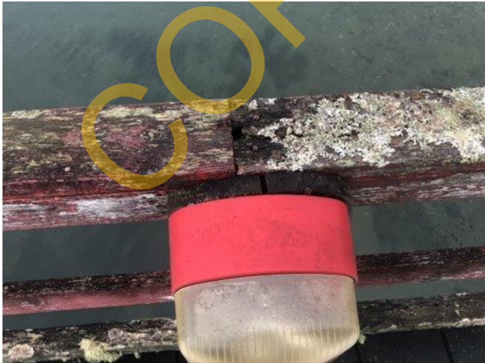
Photo 6 – Handrail deterioration between piles 8B and 9B
