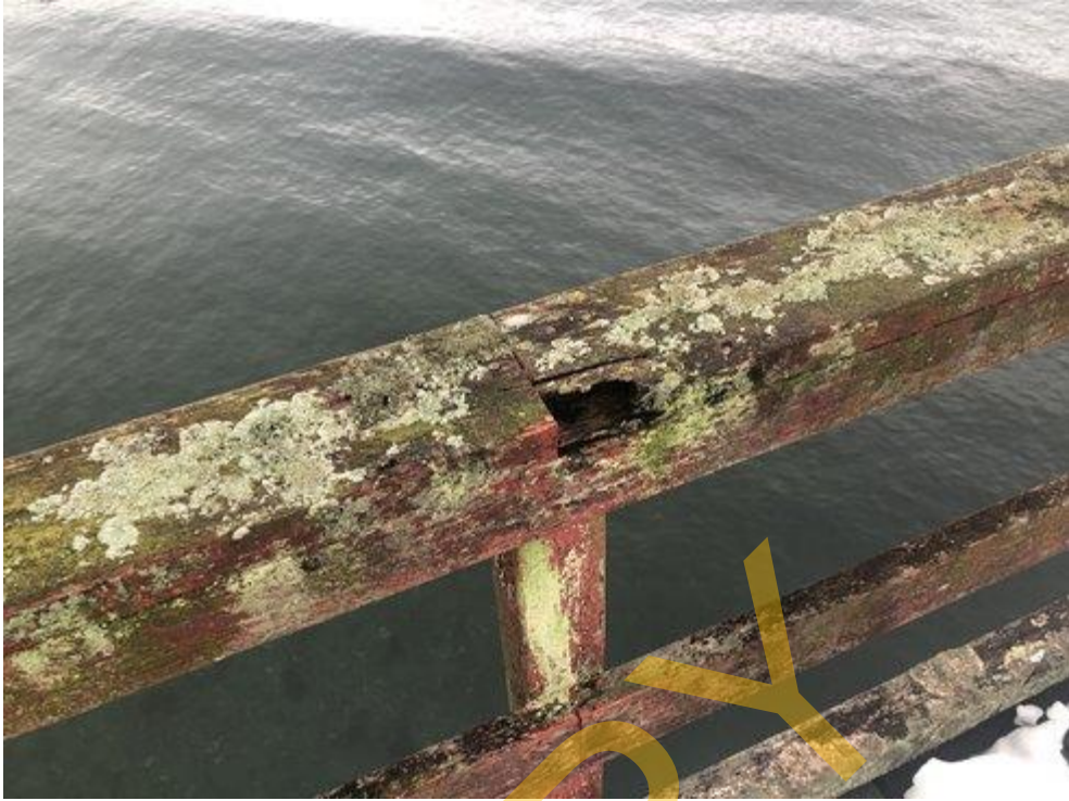
Photo 9 – Handrail deterioration between piles 12A and 13A
