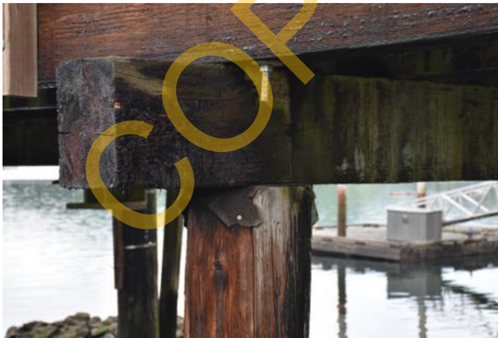
Photo 16 - Typical deteriorated capping on piles
