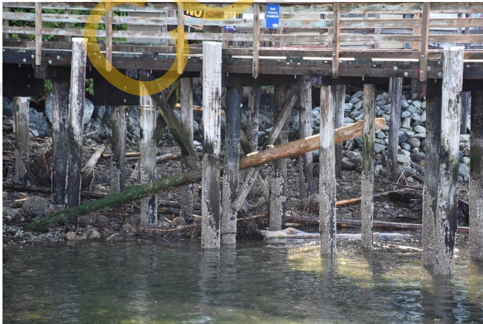
Photo 30 - North end fender piles and log debris
