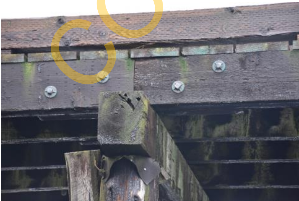
Photo 10 - Deterioration of the Pile Cap at Bent 6
