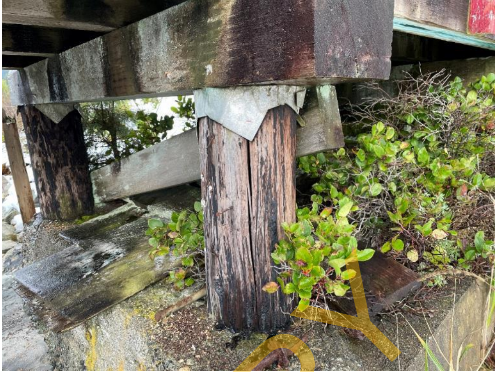
Photo 15 – Split in Pile 2A
