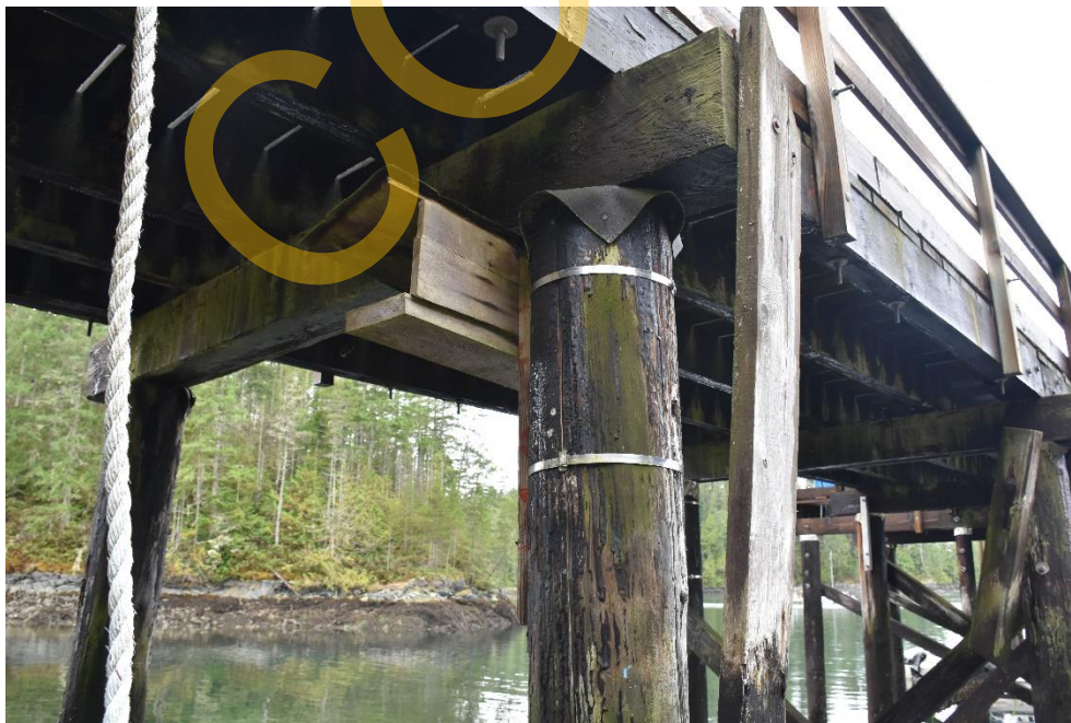
Photo 18 - Pile 5A with typical existing banded repair
