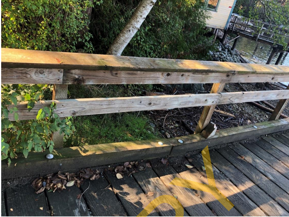
Photo 5 - Missing lower mid-rail
