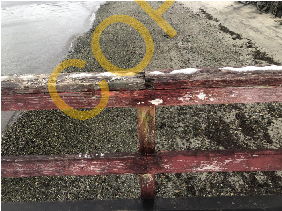
Photo 4 – Handrail deterioration between piles 4B and 5B
