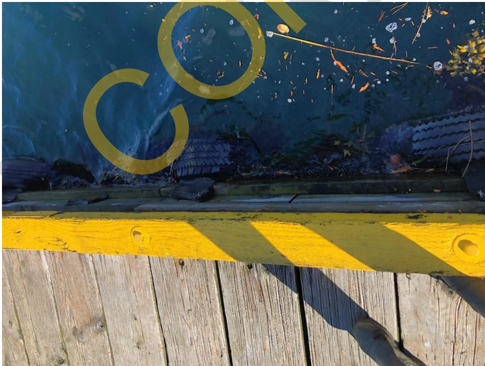
Photo 60 - Typical condition of the timber bull rails, fascia board and rubber tire fendering on the Seaplane Float
