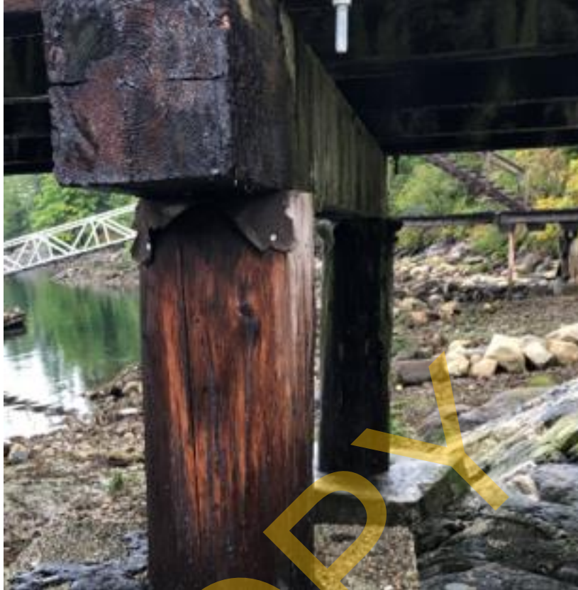
Photo 17 - Minor splitting on Pile 4B
