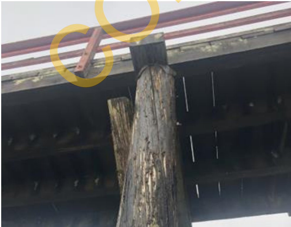
Photo 20 – Split in Pile 8A
