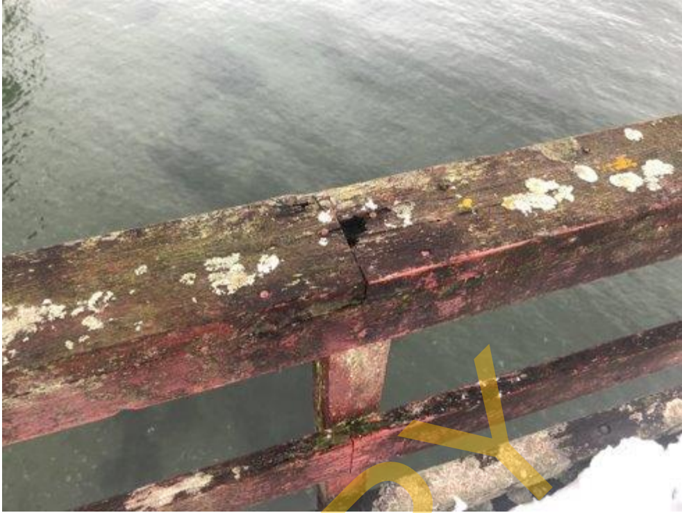
Photo 7 – Handrail deterioration between piles 9A and 10A
