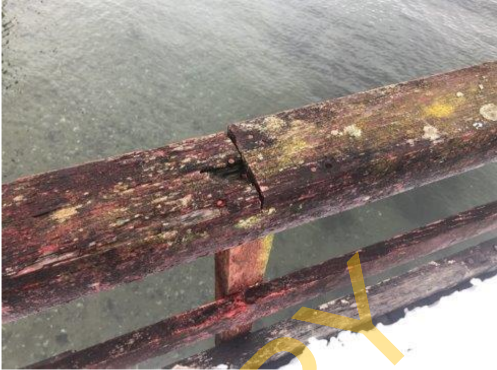
Photo 5 – Handrail deterioration between piles 7A and 8A
