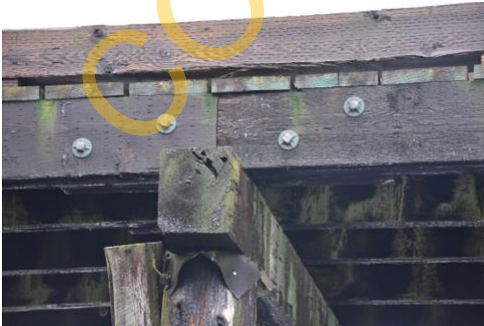
Photo 10 - Deterioration of the Pile Cap at Bent 6
