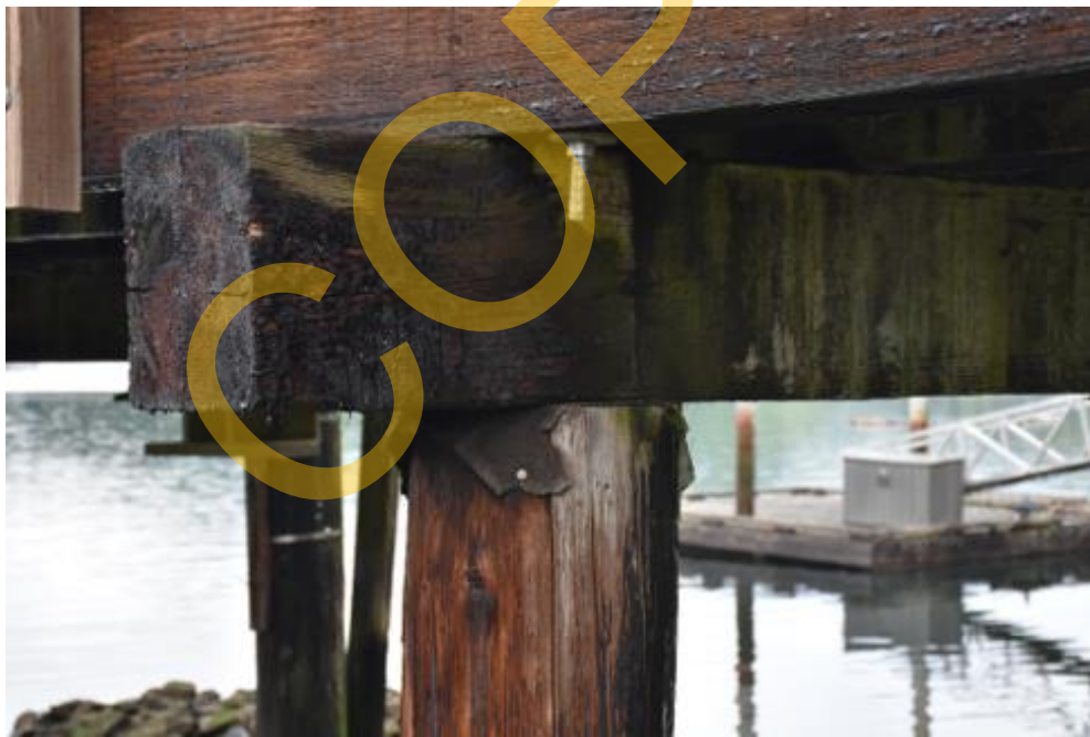
Photo 16 - Typical deteriorated capping on piles
