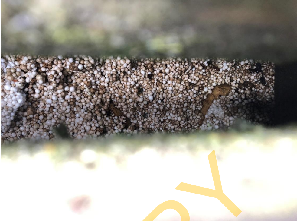
Photo 33 - Condition of exposed uncoated styrofoam billets
