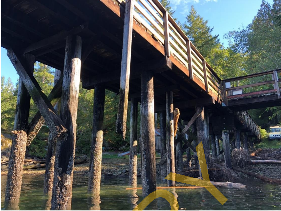
Photo 35 - Hanging side brace at pile 11B
