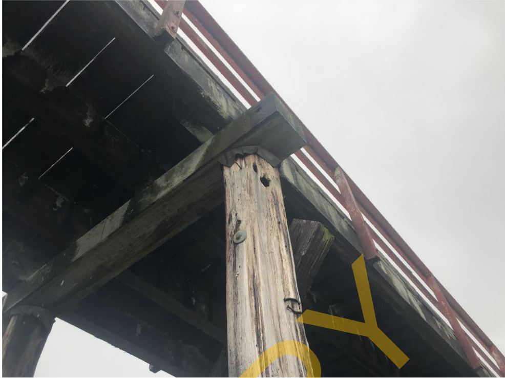
Photo 21 – Hole in Pile 9A
