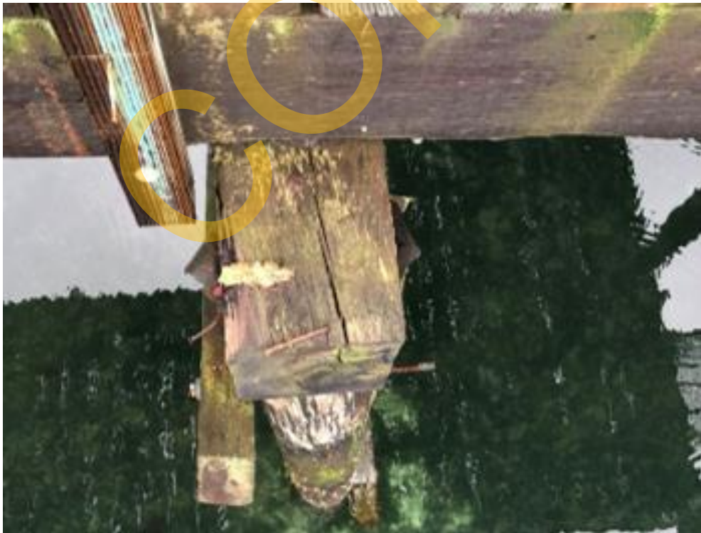
Photo 12 - Minor to moderate splitting of the Pile cap at Bent 8
