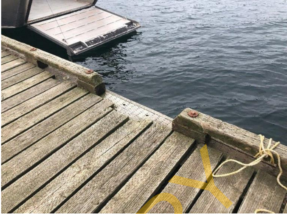
Photo 39 – Missing Bull rail on Float A
