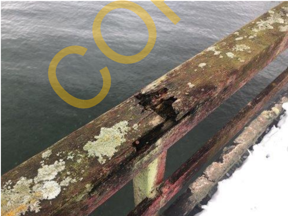
Photo 8 – Handrail deterioration between piles 11A and 12A
