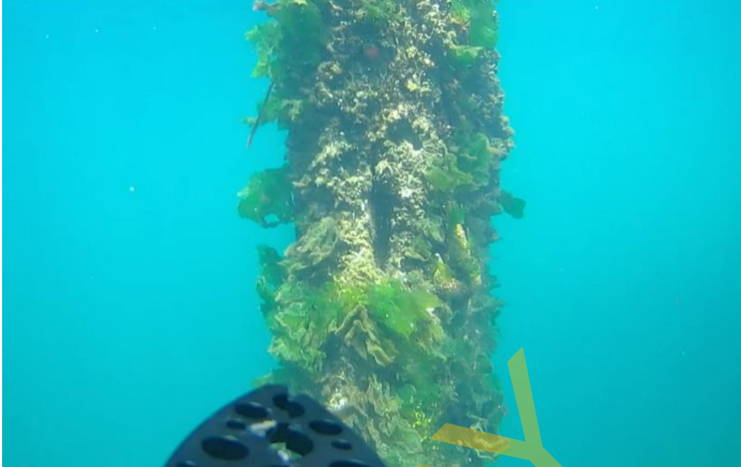
Photo 27 – Underwater image of marine borer cavity of fender pile 14A
