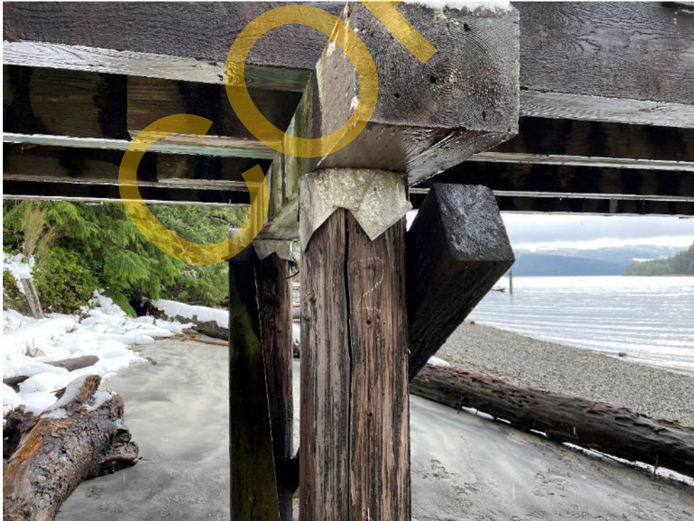
Photo 16 – Split in Pile 3B
