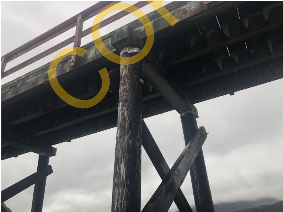
Photo 22 – Small split in Pile 10A
