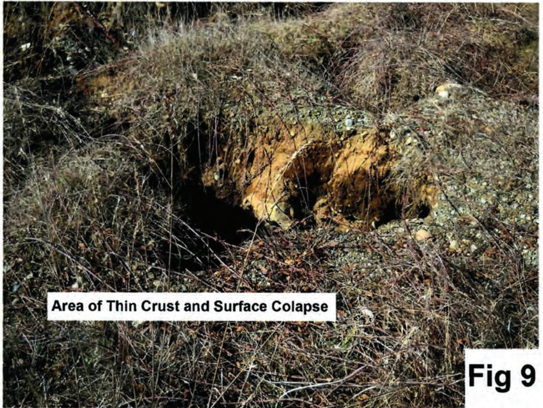
Detailed View of Surface Collapse Above Zone of Piping
