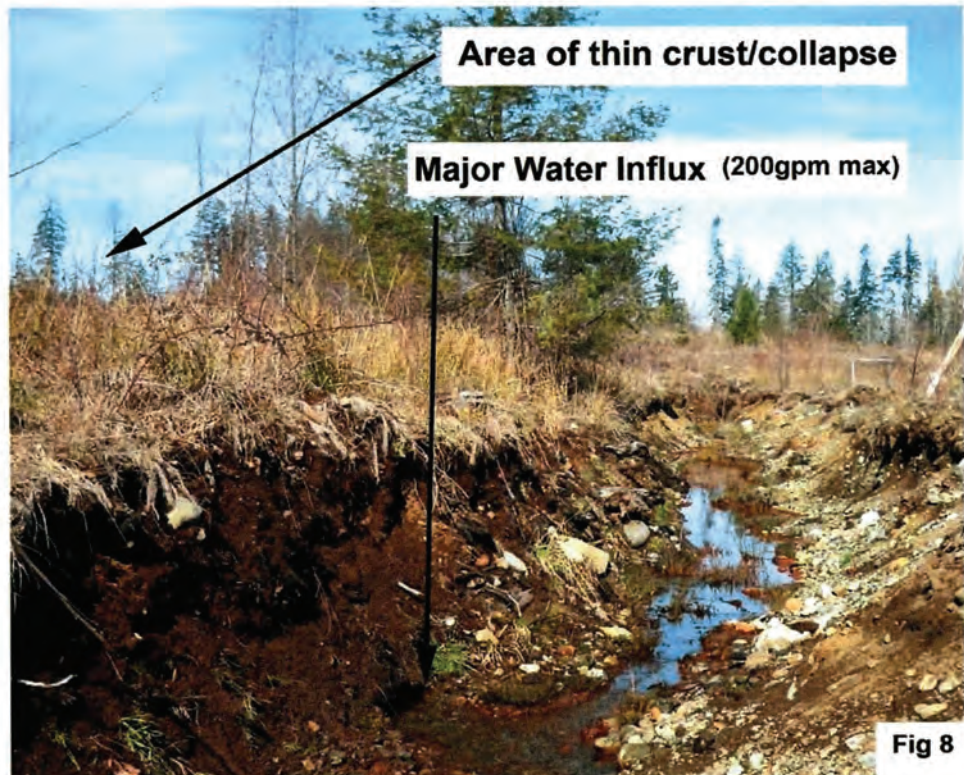
Drainage Ditch Showing Main Water Influx March 2018
