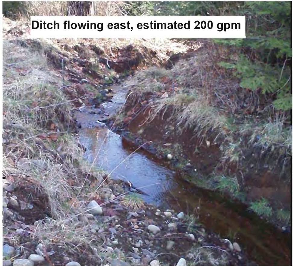
Figure 3 Ditch Draining Water Escaping by Piping at South End
