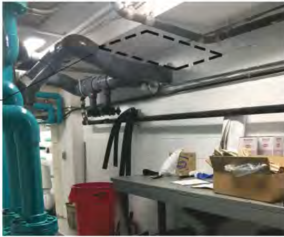
NEW PUMP TO BE LOCATED APPROX HERE. REFER TO NEW LAYOUT FOR DETAILS.
